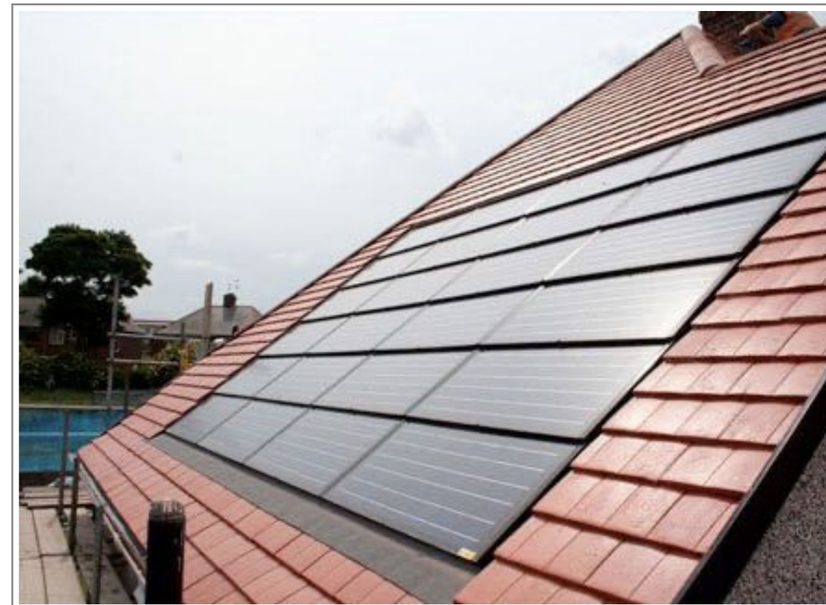
Integrated solar panels.
