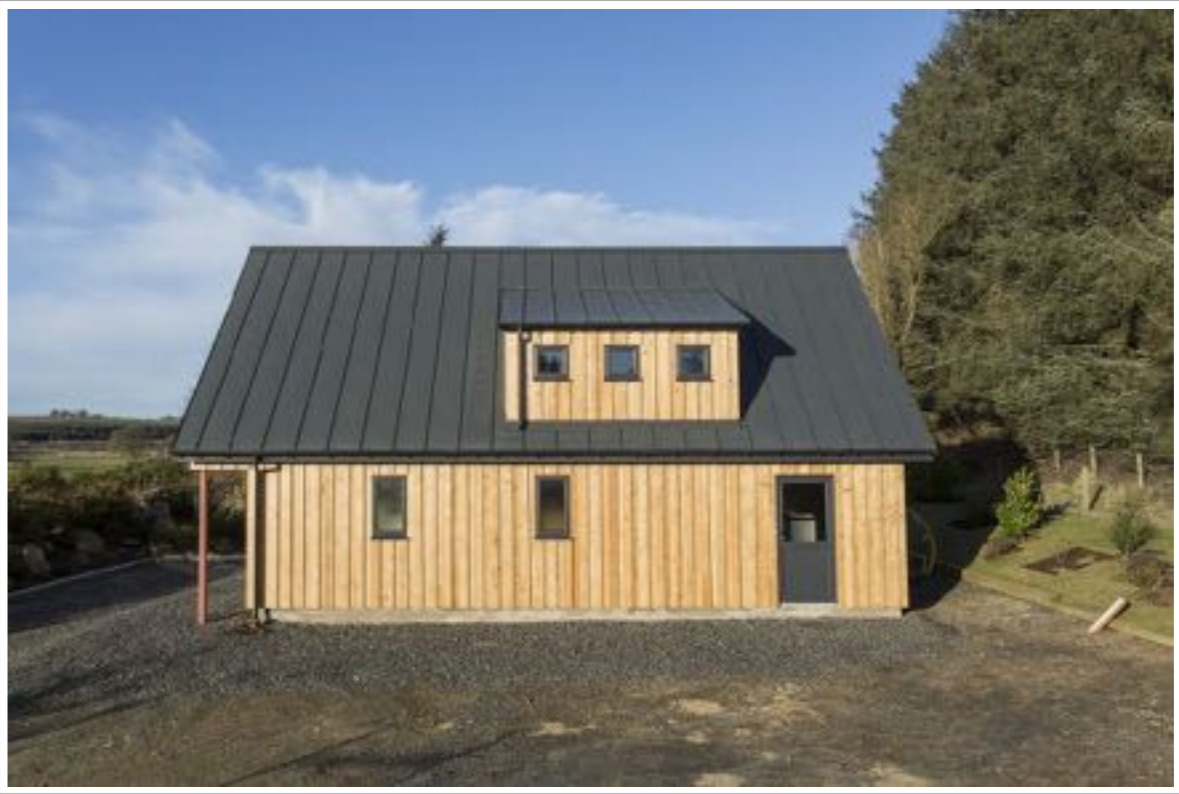
Urban Colourcoat standing seam steel panel roof in a light grey with matching rainwater goods.
