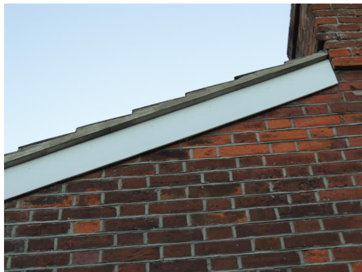
Photo 6: Showing tight seal to barge board. Note clean mortar indicating recent work to roof
