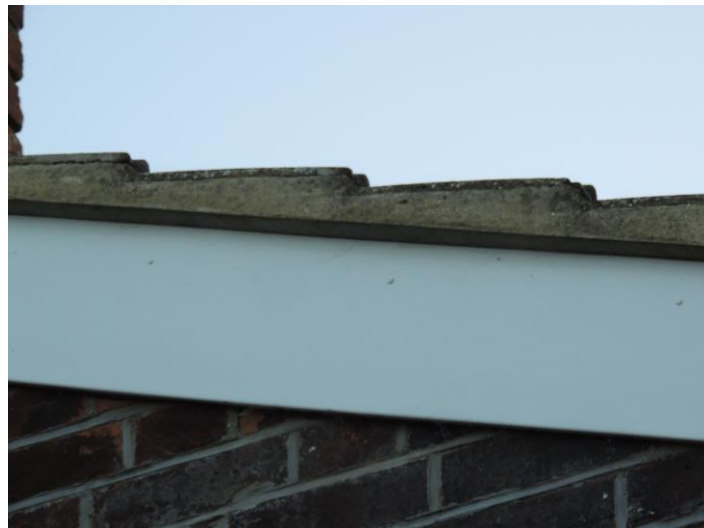
Photo 12: Showing clean mortar above barge board
