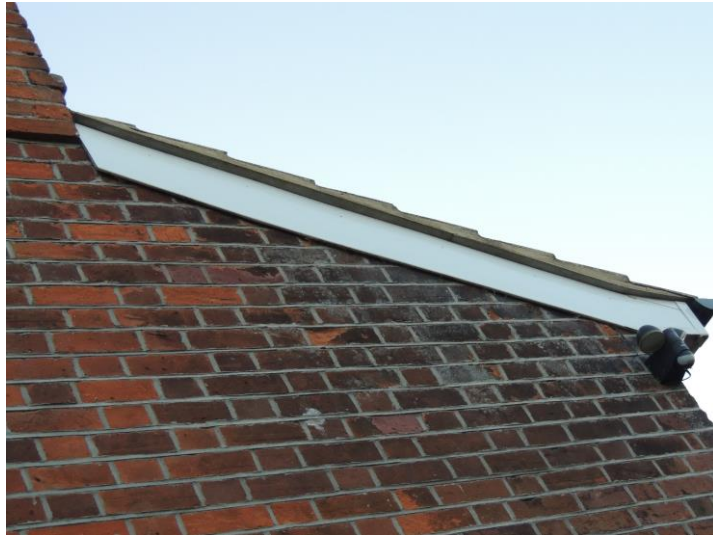
Photo 7: Showing tight seal to barge board. Note clean mortar indicating recent work to roof
