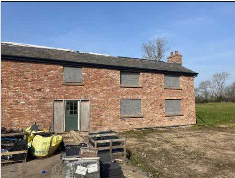
Photograph 3: A front view of the dwelling on site. The building was found with boarded windows and sections of the external roof have been removed.
