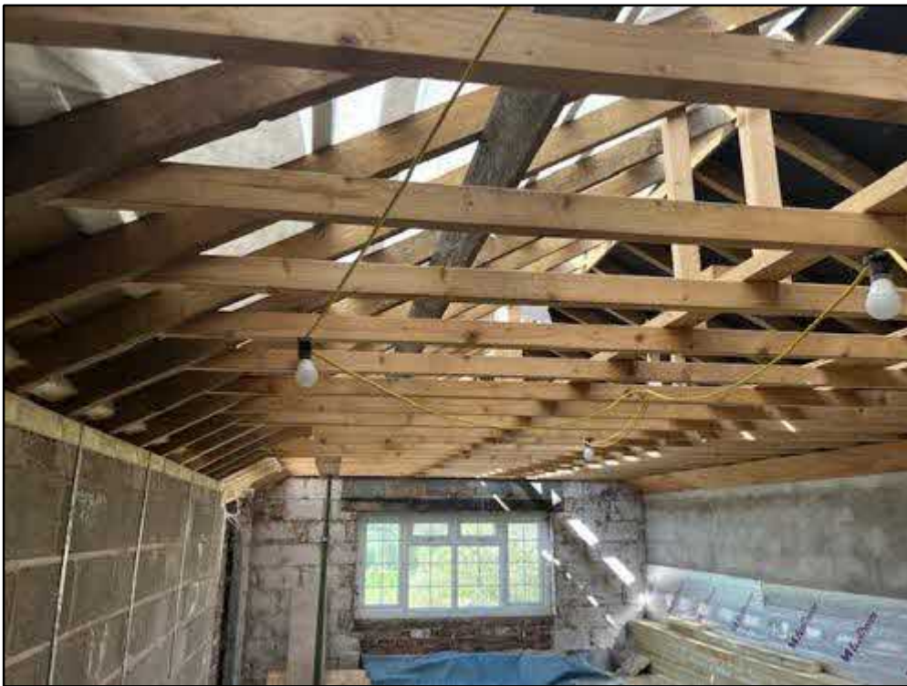
Photograph 12: An internal view of the first floor of the building. The roof space has been stripped back in places, as a renovation on the previous dwelling has been abandoned.
