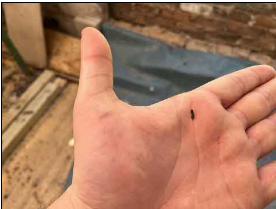
Photograph 13: Droppings found on the first floor.
