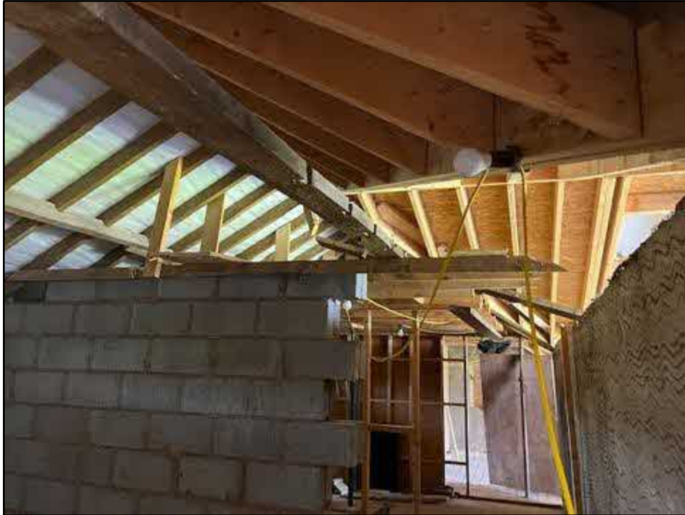
Photograph 13: Another view of the internal roof space. Large openings have been created by wall demolition.
