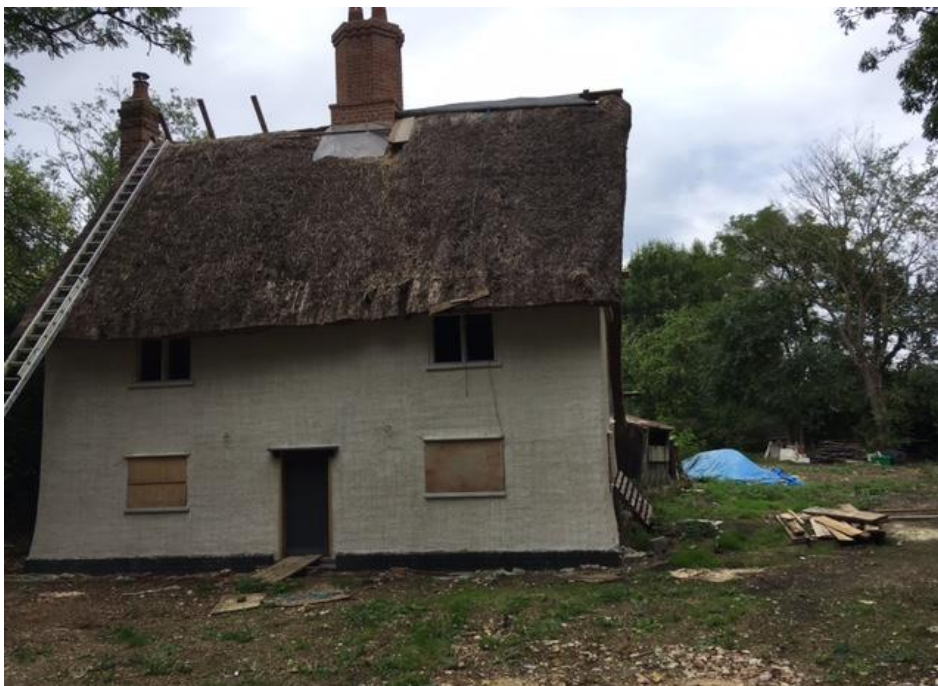
Front of The Cottage as viewed from Broad Green Lane (repair work on-going)
