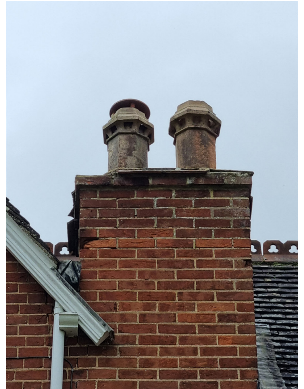
Existing decorative pots to be retained. Sections of deteriorated brickwork and flaunching to be repaired.
