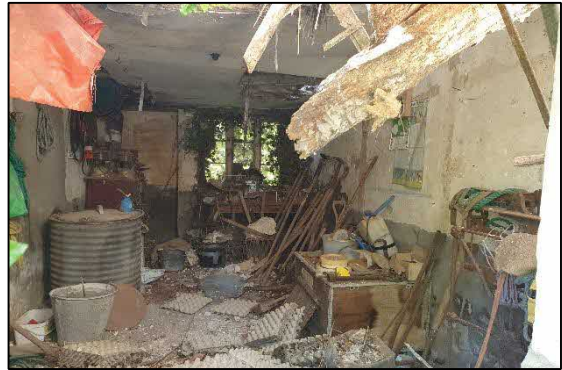
Figure 5: Room 2 – collapsed ceiling
