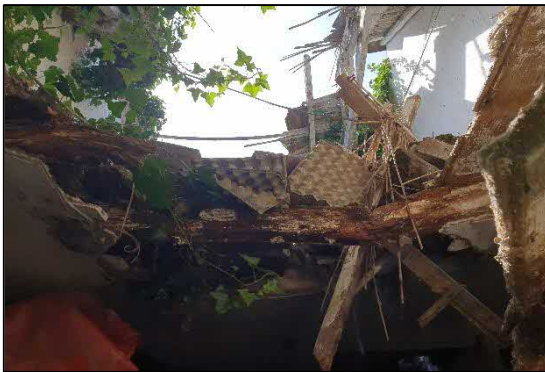
Figure 6: Room 3 collapsed roof.
