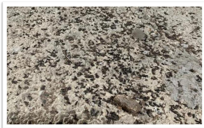
Figure 6: Large numbers of bat droppings were present under most mortice joints in the barn.
