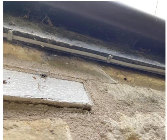
Photo 10, "Gaps under the wooden fascia"
