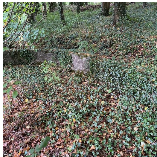
Plate 4: View of retaining wall around existing gravel parking area that will have restricted root growth of adjacent trees.
