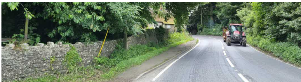
Fig 5. View of the existing boundary wall adjacent to the A37. Part of the wall is proposed for raising and incorporation into the proposed extension
