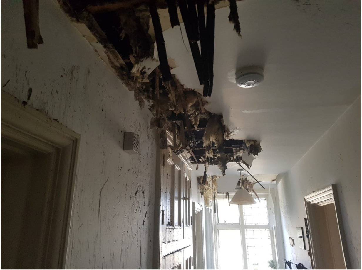
Above: photograph showing the extend of the damage to the hall of the apartment No.10.
