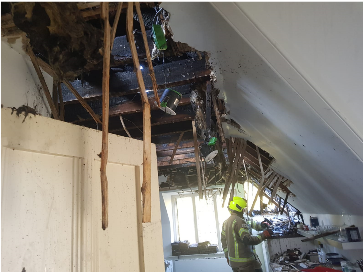
Below: photograph showing damage to the kitchen of the apartment 10. This was the origin of the fire.
