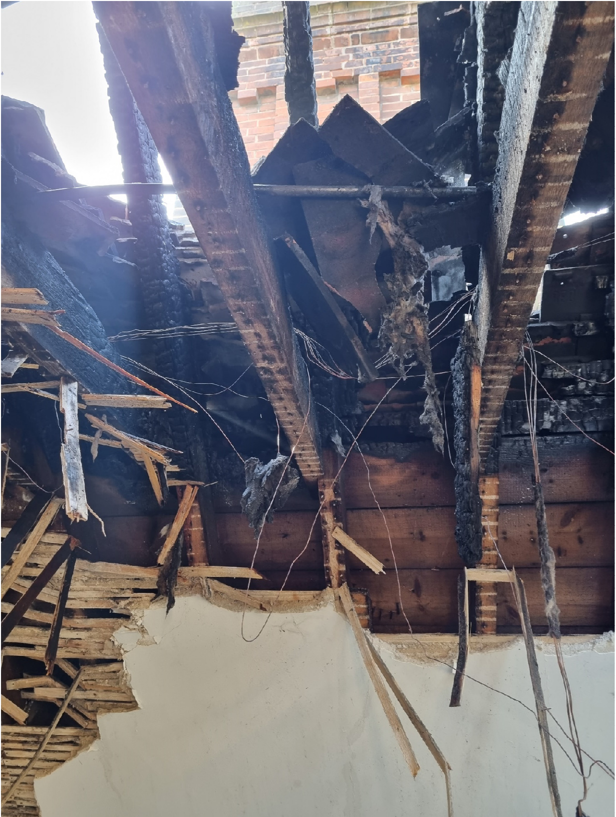
Above: kitchen of the apartment No.10. The location of the origin of the fire.
