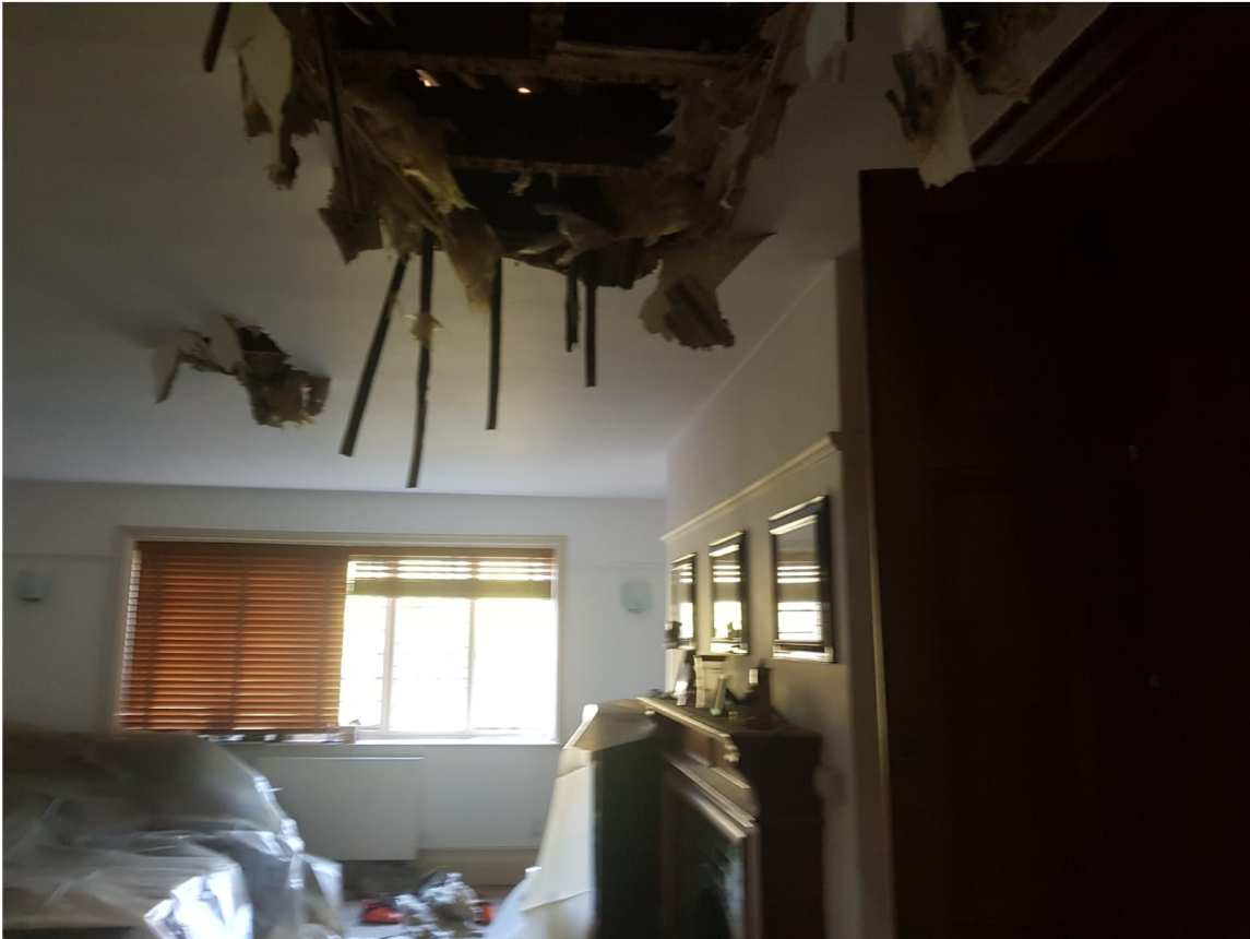
Above: fire damage to the apartment 10 living room.
