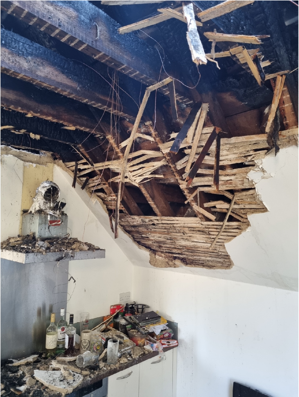
Above: photograph showing damage to the kitchen of the apartment 10.
