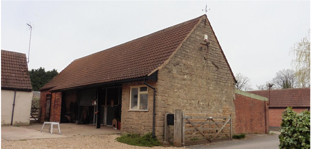
Photograph 2: South aspect and east gable of outbuilding at Abbeyfields Farm, Newstead Abbey Park
