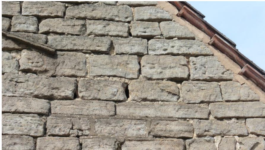
Photograph 6: East gable with gaps in stonework due to erosion of mortar
