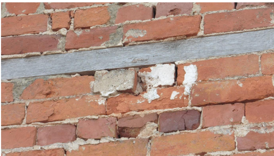
Photograph 7: West gable with deteriorating mortar in brickwork and gaps around timber lintel
