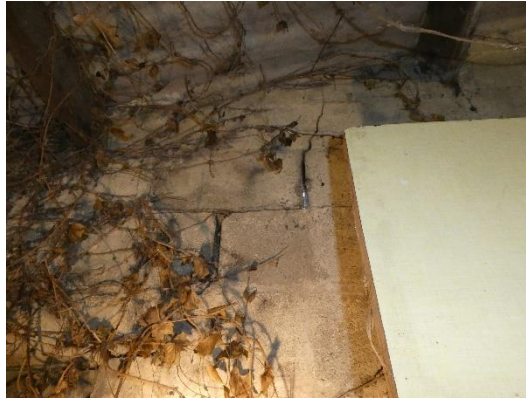
Photograph 21: Gap in blockwork wall that extends to the exterior
