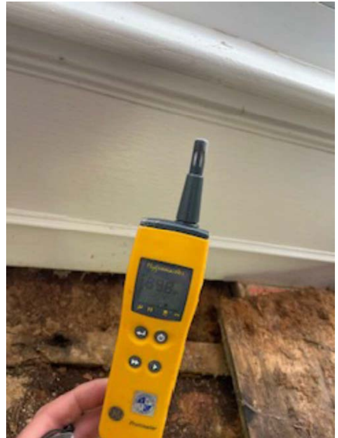
HYGROMETER SHOWING SUB-FLOOR HUMIDITY
