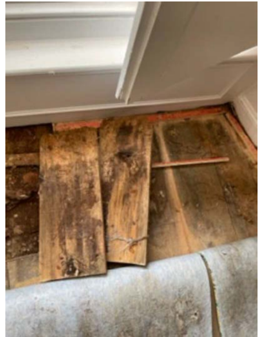
SHOWING FUNGAL MATERIAL ON UNDERLAY AND FLOORBOARDS.
