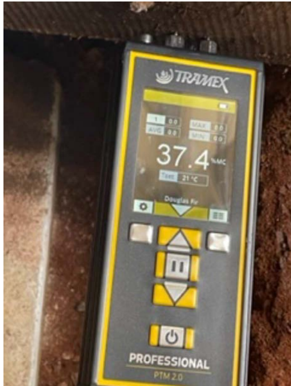
SHOWING HIGH MOISTURE READINGS.
