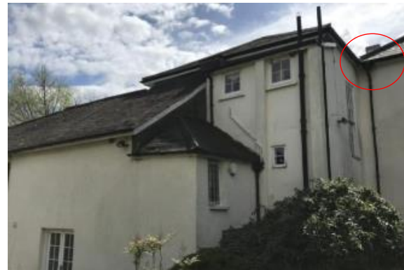
Plate 2. Northern elevation where Tudor section meets Georgian section. Location of serotine emergence shown in red.
