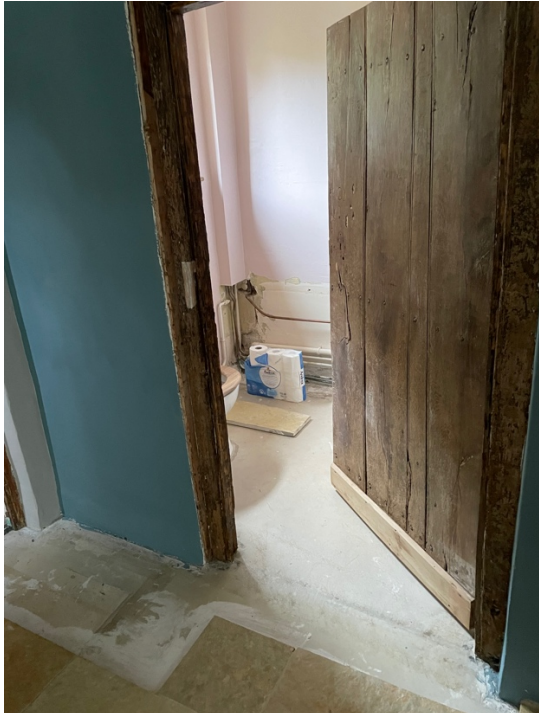
Photo 3.8. Bathroom (WC on floorplan). Note original floor after stripping carpet of levelling compound over concrete, floor tiles and stripped door and frame.
