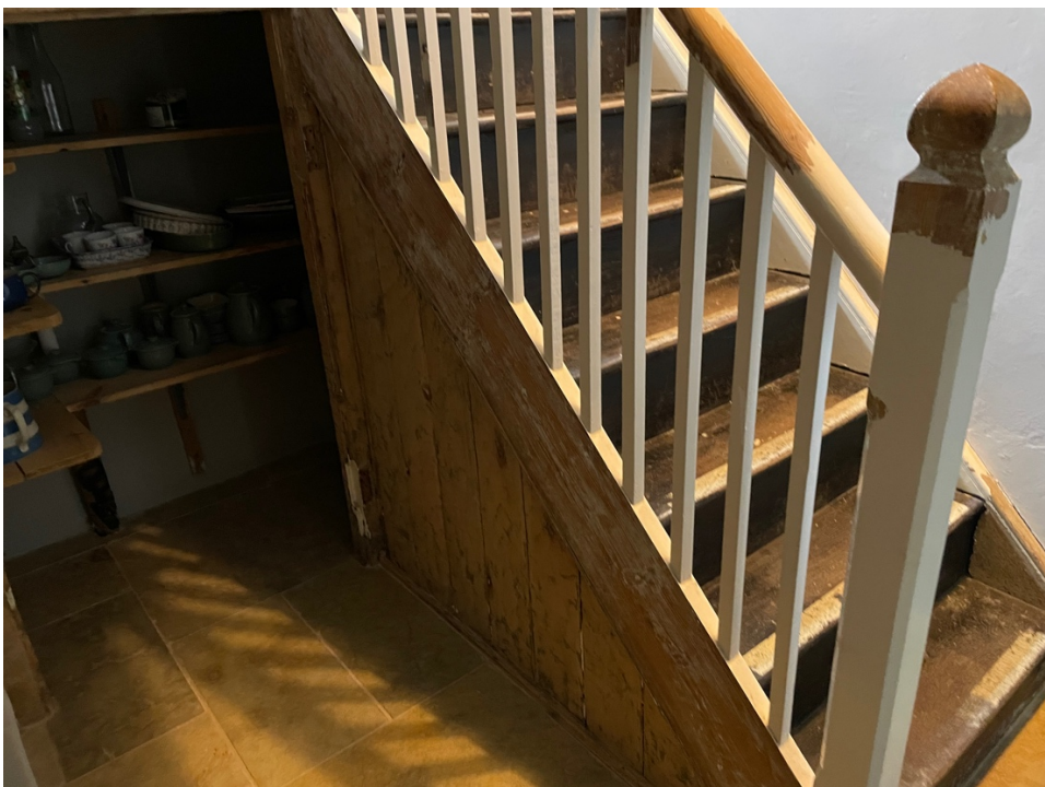
Photo 3.7. Back staircase. Note staircase part stripped of gloss paint and the new stone tiles.
