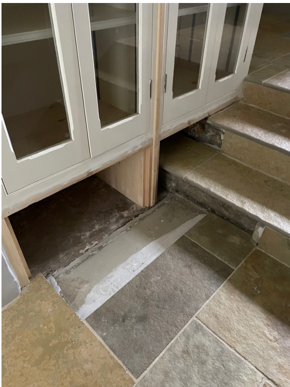
Photo 3.3. The built in cupboards on the back corridor near the step (refer to floorplan). Note the original concrete/levelling compound floor that was found under the carpet.
