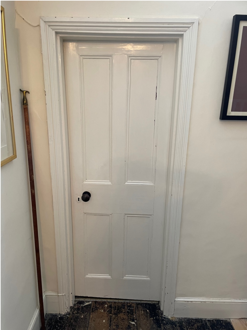
Photo 3.10. Door to bathroom from landing on first floor – gloss painted pine to be stripped
