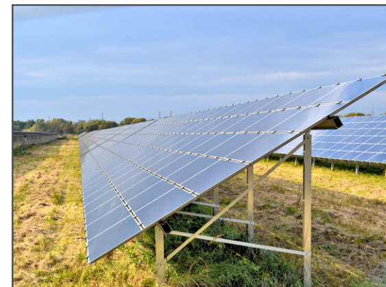
Plate 4 - Typical Solar Array and Panel Frames with Anchors
