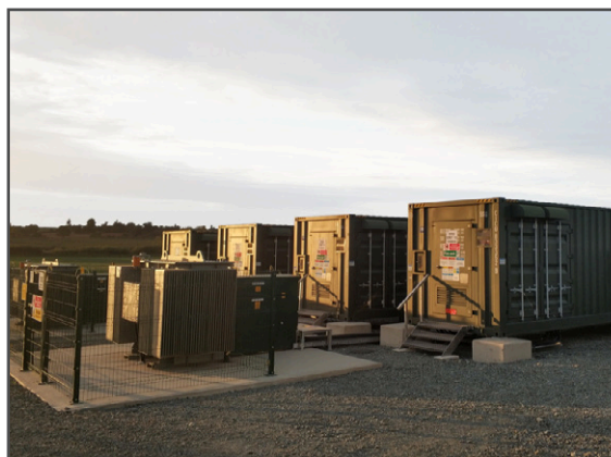
Plate 12 - Typical Battery Energy Storage
