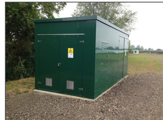
Plate 8 - Typical Transformer equipment
