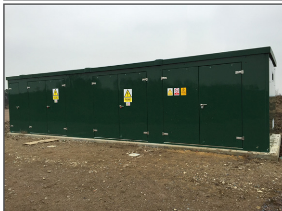
Plate 13 - Typical Substation Units - examples of brick and GRP finish
