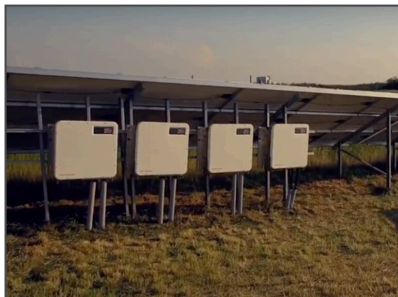
Plate 7 - Typical string-inverter units
