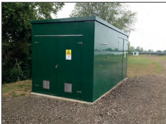
Plate 12 - Typical Transformer equipment
