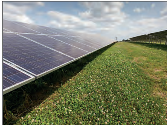
Plate 9 - Typical Solar Array
