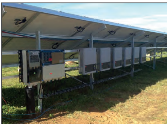
Plate 11 - Typical string-inverter units
