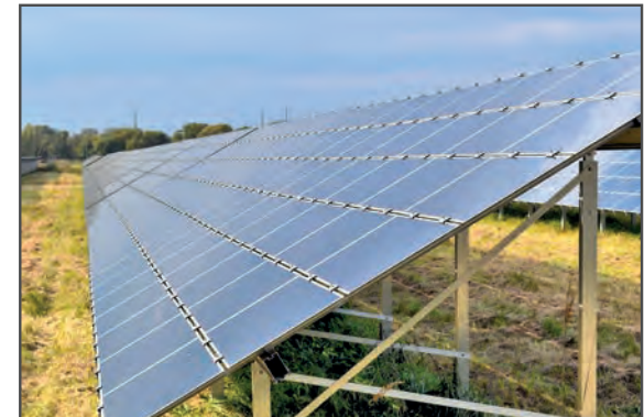
Plate 1 - Typical Solar Array
