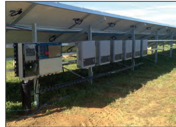
Plate 3 - Typical String Inverter Unit
