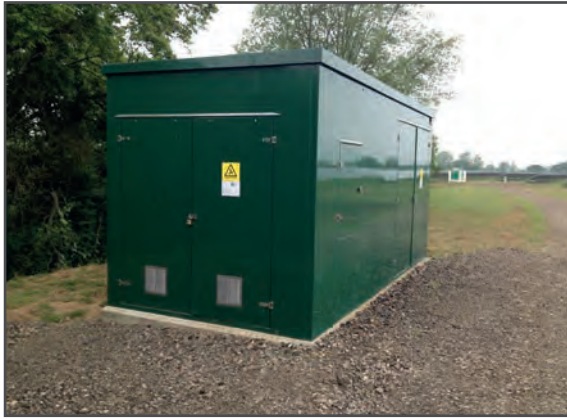
Plate 4 - Typical Transformer Equipment
