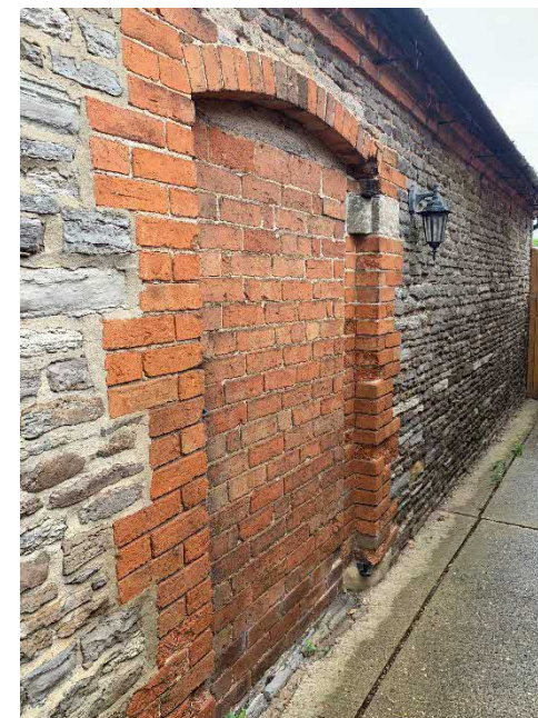
Photo 15: Blocked up structural opening
