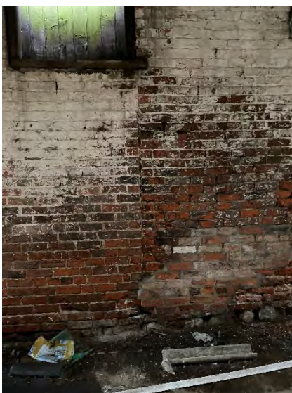
Heavily eroded brickwork
