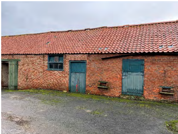
Dilapidated Rainwater goods
