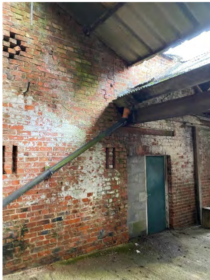
Defects around ventilation holes
