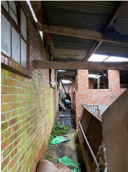
Poor roof construction
