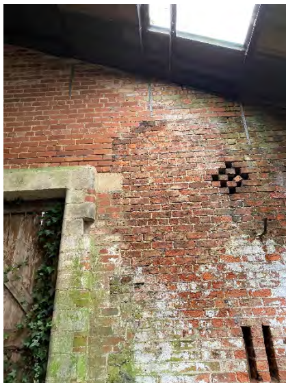
Defects around ventilation holes
