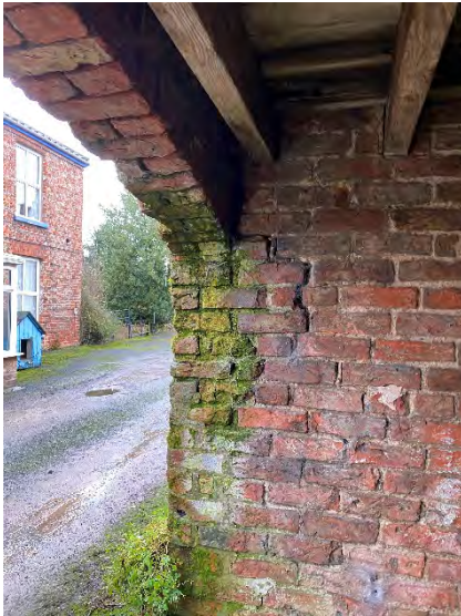
Movement around arch
