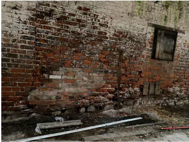
Heavily eroded brickwork
