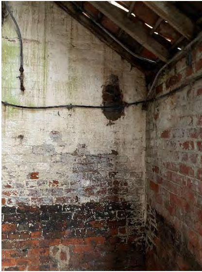
Dilapidations of Roof
