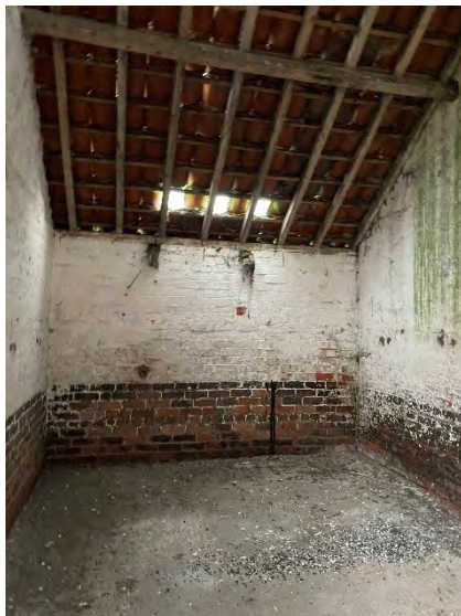
Dilapidations of Roof
