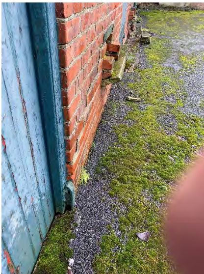
Lateral movement/damage to West Elevation
