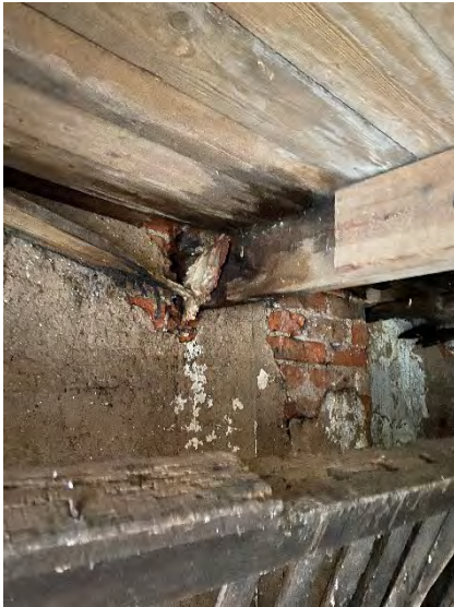
Defects in timber partially rectified
