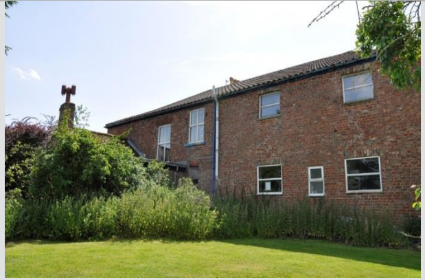
Plate 30: Garden facing elevation with irregular fenestration, all UPVC window units and flat roof extension to the 20 th century extension to the sitting room
