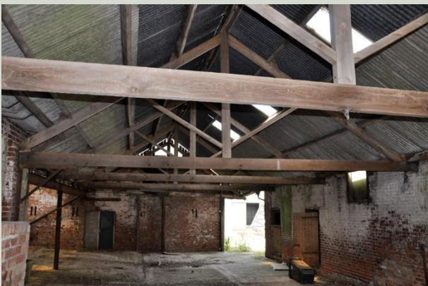
Plate 41: The eastern part of the covered yard area is formed from timber king post trusses attached to the brick walls of existing buildings and set on posts with a corrugated sheeting dual pitched roof
