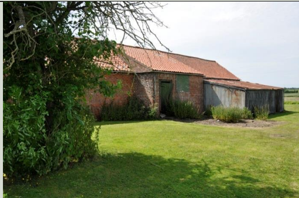
Plate 6: The stalls project to the rear elevation where there is a poor quality structure formed from corrugated sheeting
