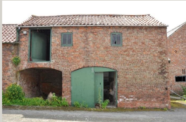
Plate 13: Northern bays of the barn are two storey with first floor taking-in door and windows facing the access track and stores below
