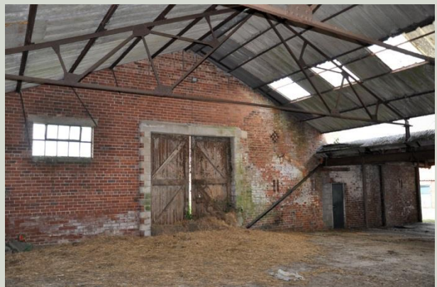
Plate 42: The covered yard that forms the northern yard to the piggery has a modern metal portal-framed roof structure with corrugated sheeting dual pitched roof cover
