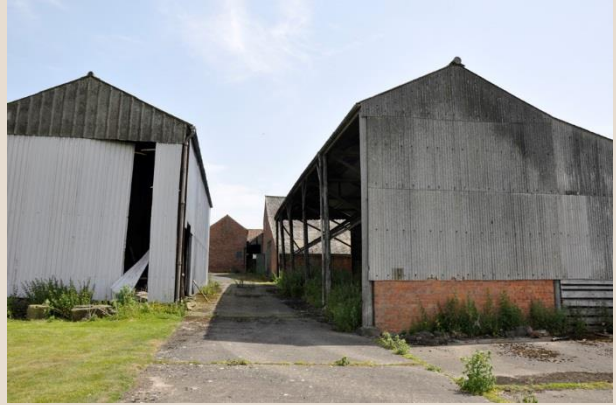
Plate 44: Looking south towards the north ends of both sheds, open fronted elevation to cattle shed is apparent
