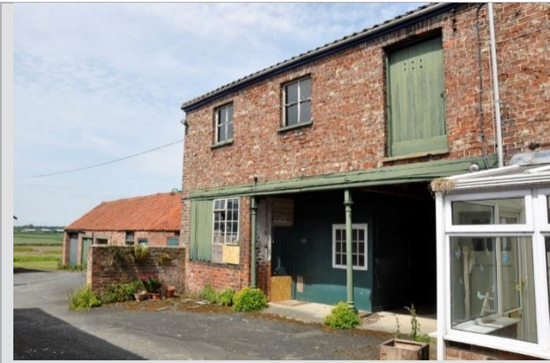
Plate 33: Northern bays to the house have a more agricultural character and appearance
