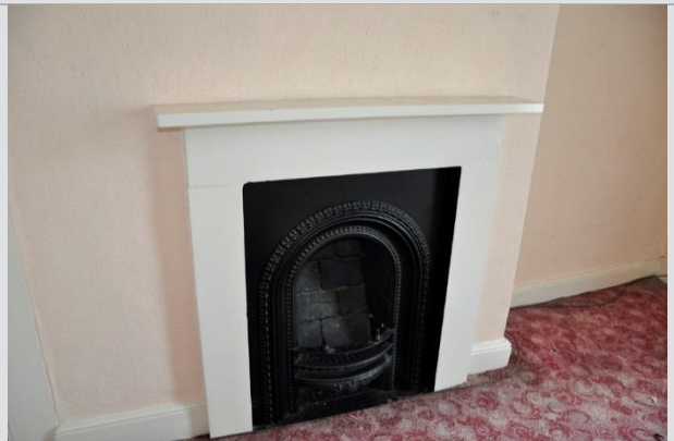
Plate 32: Late Victorian style round arched cast iron fireplace to a first floor bedroom
