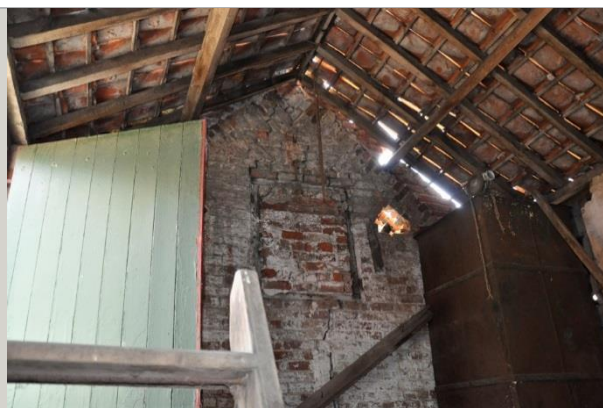
Plate 17: Blocked hayloft opening in south gable of two storey range and evidence that the roof has been rebuilt
