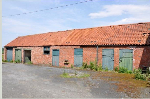
Plate 5: The end three bays are likely former tack / harness rooms and stores
