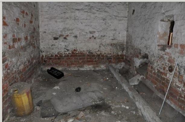
Plate 15: Northern bay is an animal loose box with low level feeder and trough i.e. for pig or calf use
