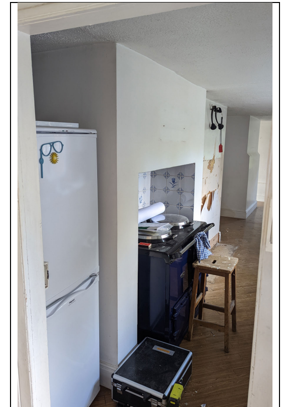
Permission is sought of removal of part of the "Aga chimney" breast.
