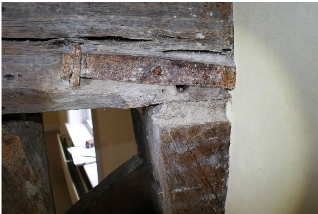
C18th wrought iron tie used to repair the failed joint in the top-plate. Looking E.
