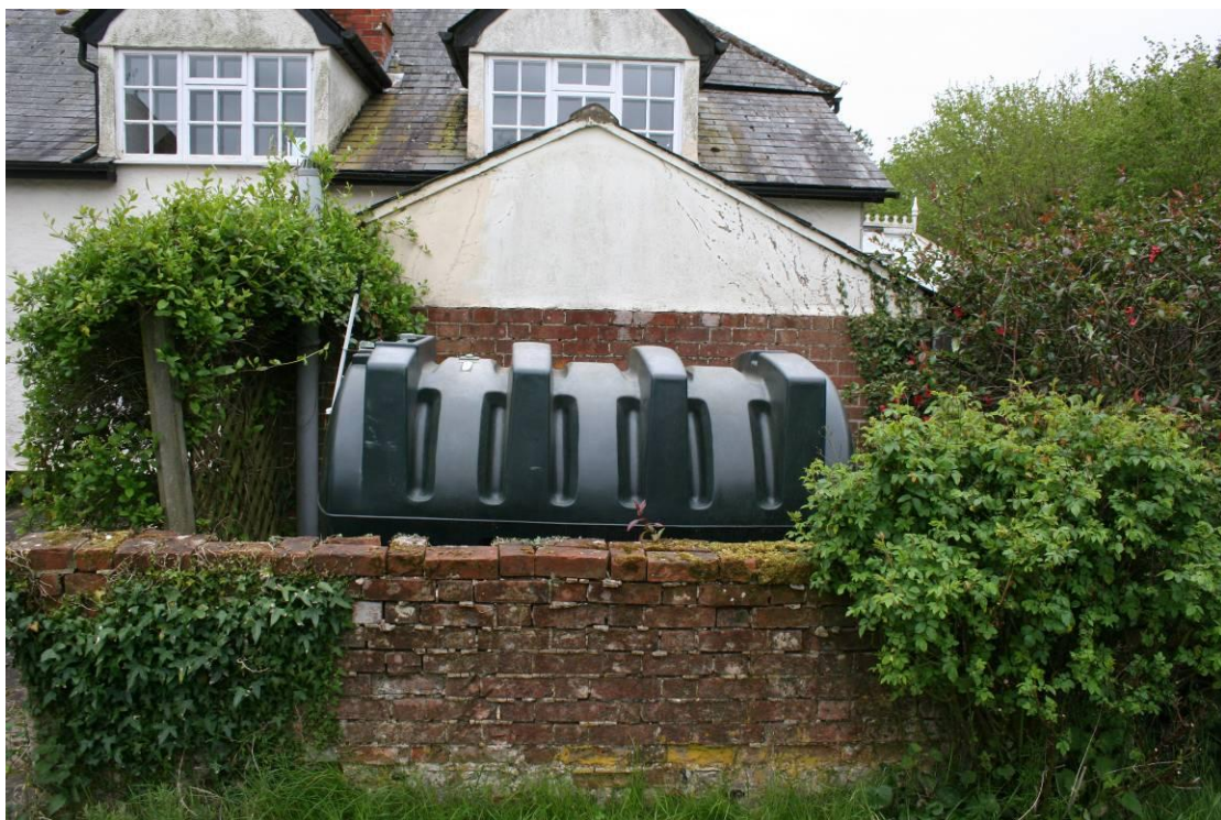
The north elevation of the Outshot is partly hidden by a plastic oil tank.
