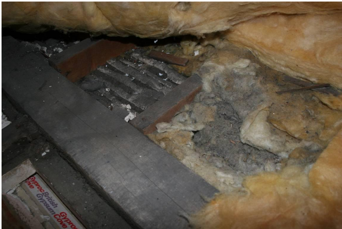
Earlier softwood main ceiling joist with skew nailed common joists. Note plasterboard.
