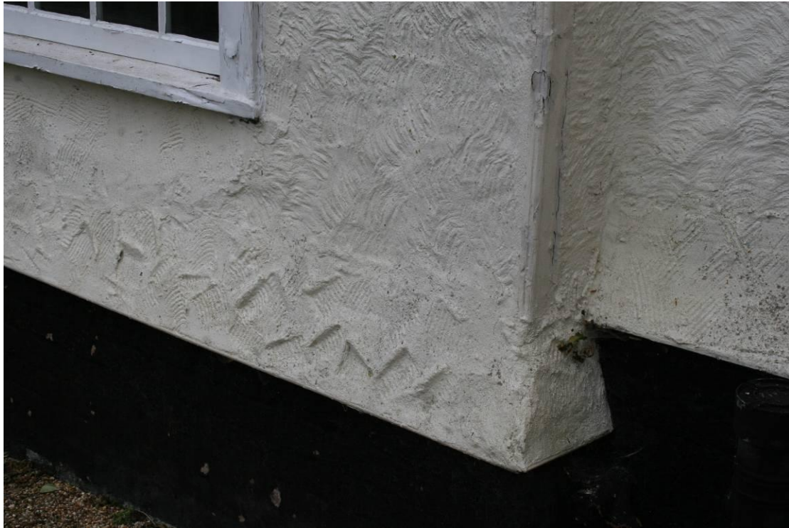
Detail of the modern render and galvanised drip detail on the NE corner.
