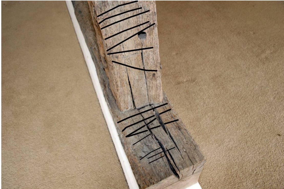
The storey post has a slip tenon which is numbered to match the sole plate.
