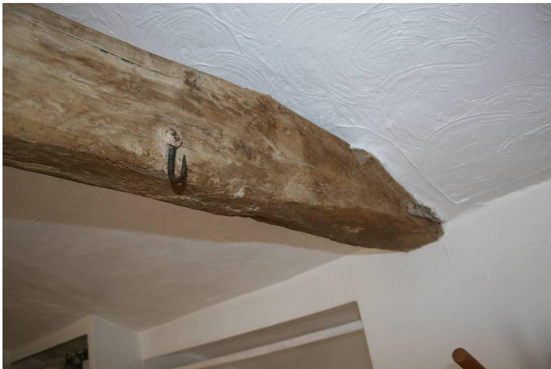
The western end of the tie-beam with short iron tie and carcase hook.
