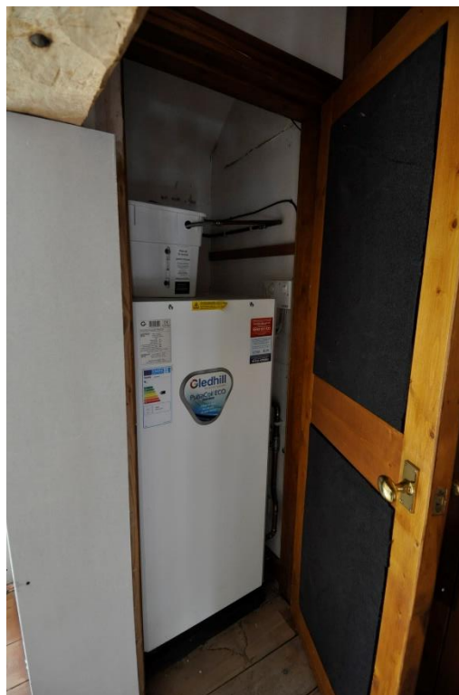
Services cupboard in west bedroom
