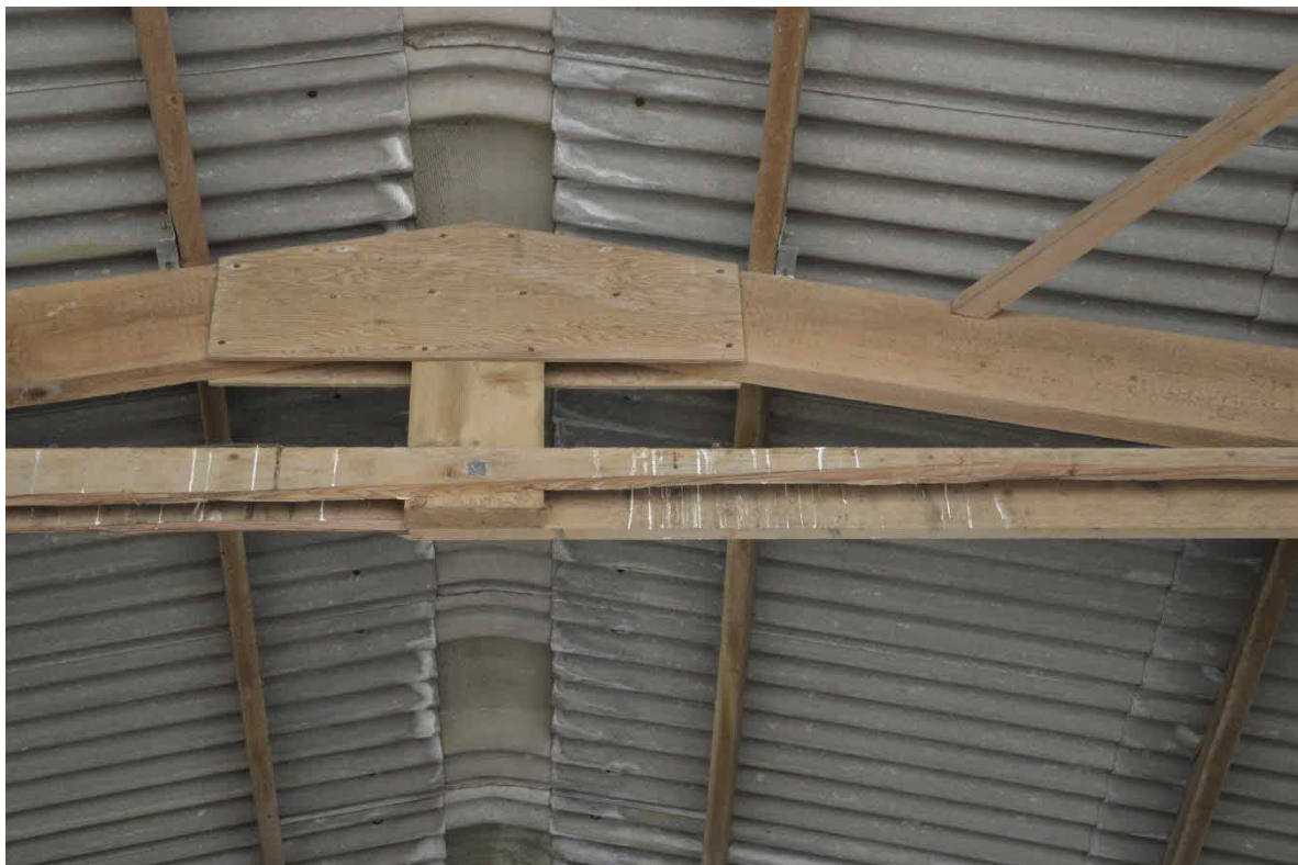
Plate 12. Evidence of roosting barn owl on roof timbers 2019
