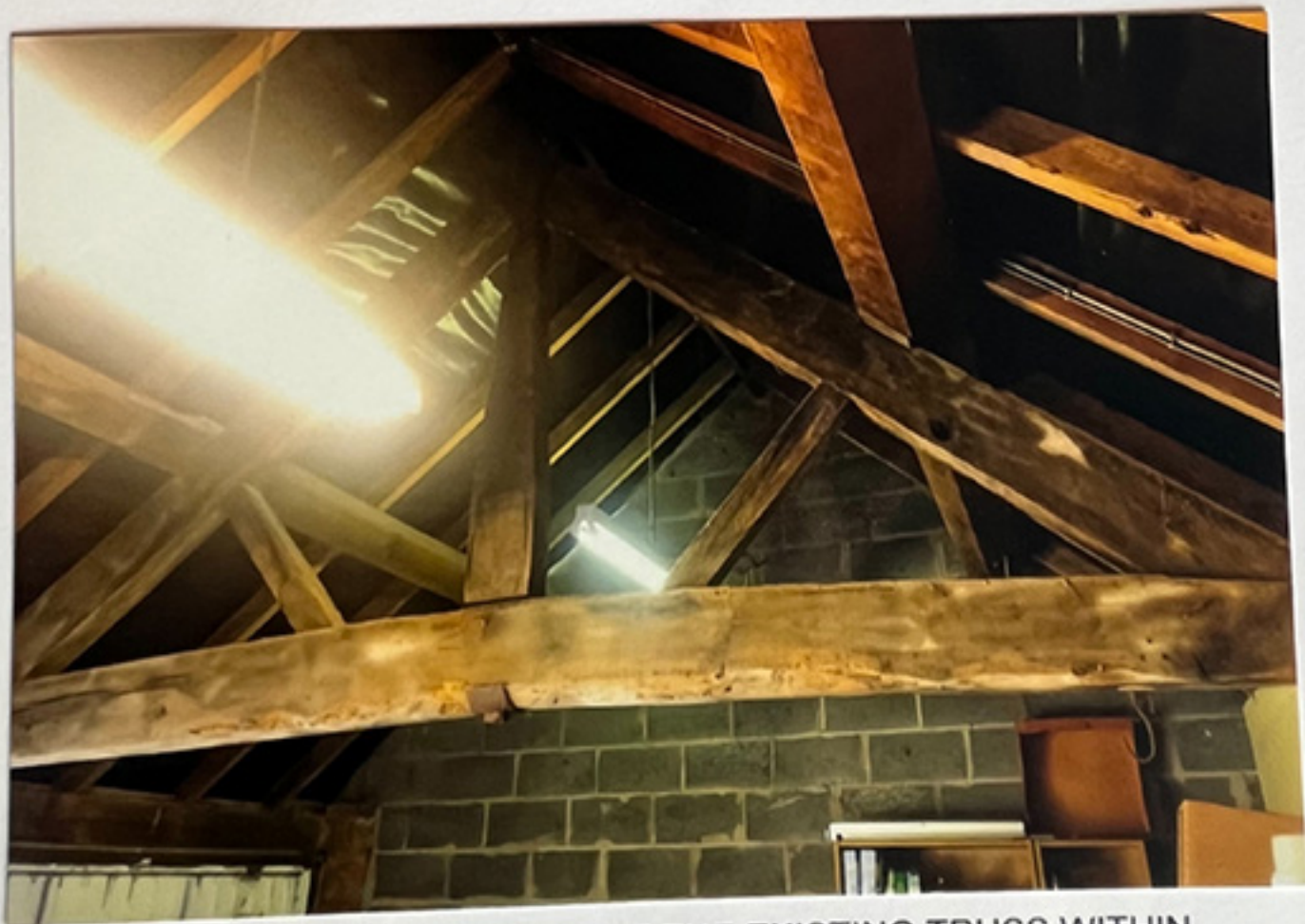
PHOTOGRAPH 5 - DETAIL OF THE EXISTING TRUSS WITHIN THE GARAGE BAYS. THIS WOULD BE VISIBLE WITHIN THE PROPOSED UTILITY ROOM AFTER THE PROPOSED WORKS.
