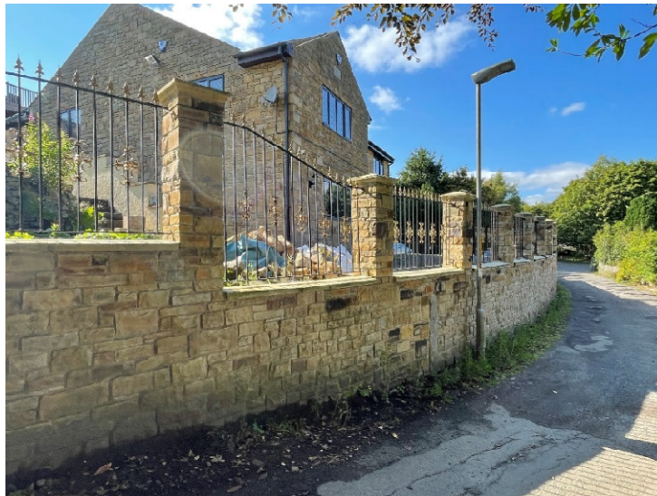
View of retaining wall with new pillars and rails looking down Mill Lane
