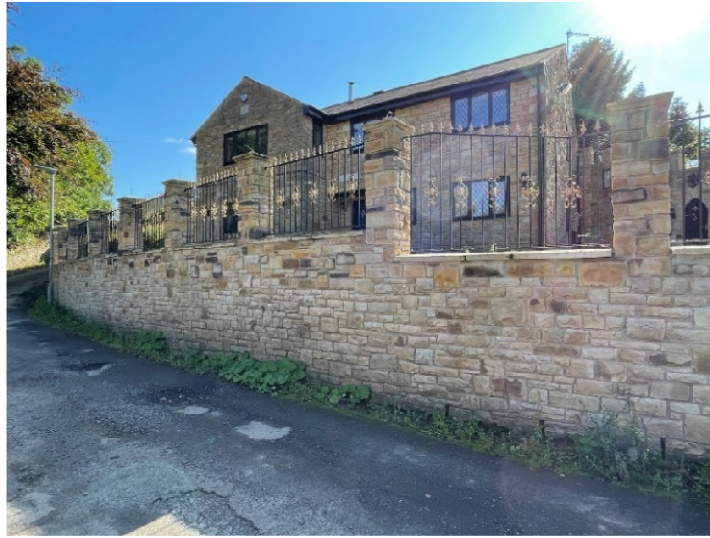
View of retaining wall with new pillars and rails looking up Mill Lane
