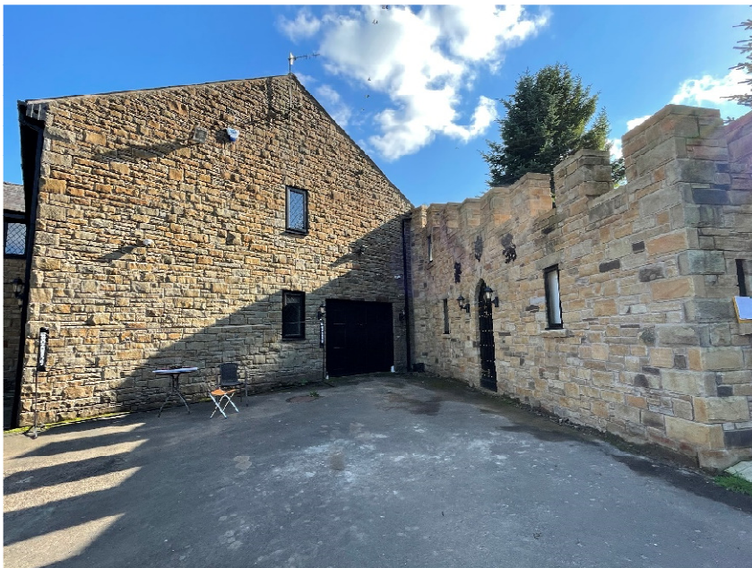
Street view of wall to rear yard/steps after facing in stone, facing commenced Sept 2021 and completed Oct 2021
