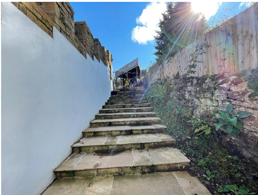
Photograph of rear of wall showing existing rendered wall acts as a retaining wall and protection to fall from steps rising up.
