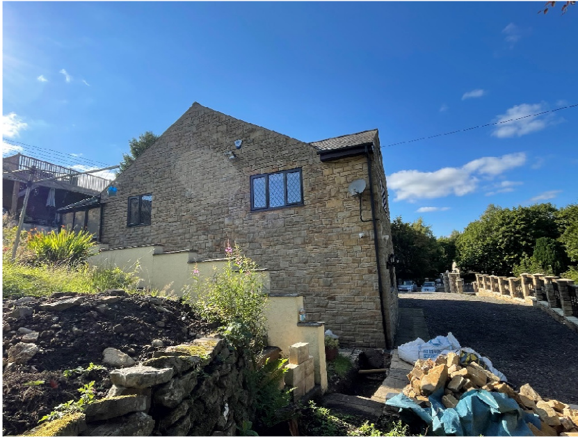
Shows level of ground behind boundary wall outside house and the newly constructed piers and fence to protect against fall
