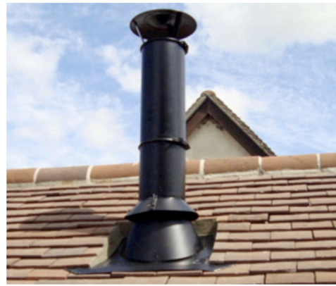
Roof Mounted Woodburning stove Flue (Black twin wall)
