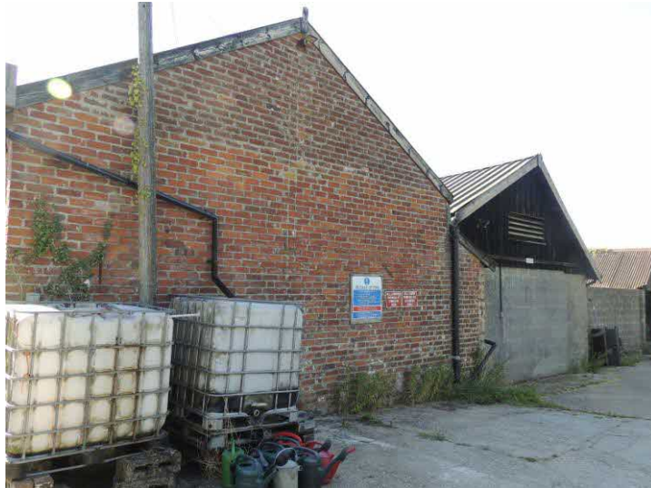
Photo 7: Two single-storey, pitched roof buildings attached to the western side of the barn are unaffected by the project.
