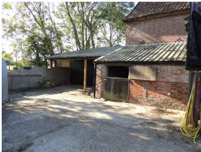
Photo 9: A garage and shed at the western end are unaffected by the proposal
