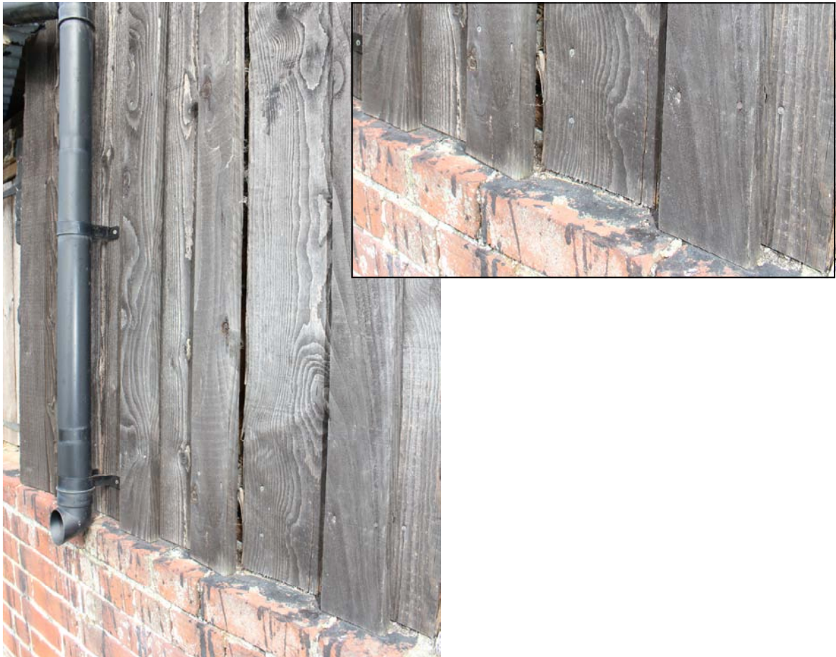
Fig. 32: Detail of overlapping plank framing of south gable of east shelter shed
