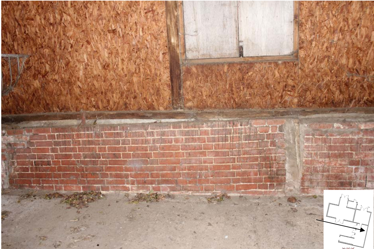
Fig. 26: Rear dwarf brick foundation wall of east shelter shed in monk bond
