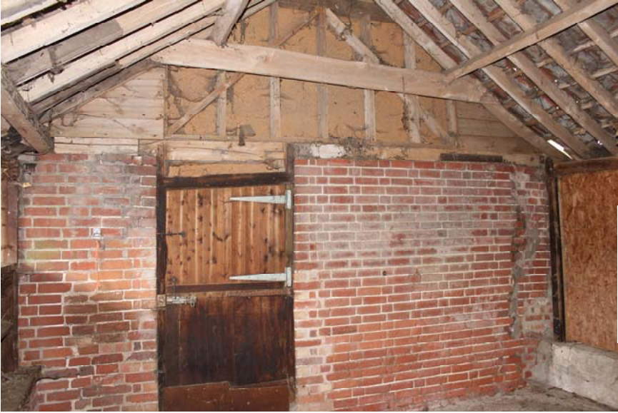
Fig. 28: South face of rear wall of east single storey room viewed from shelter shed
