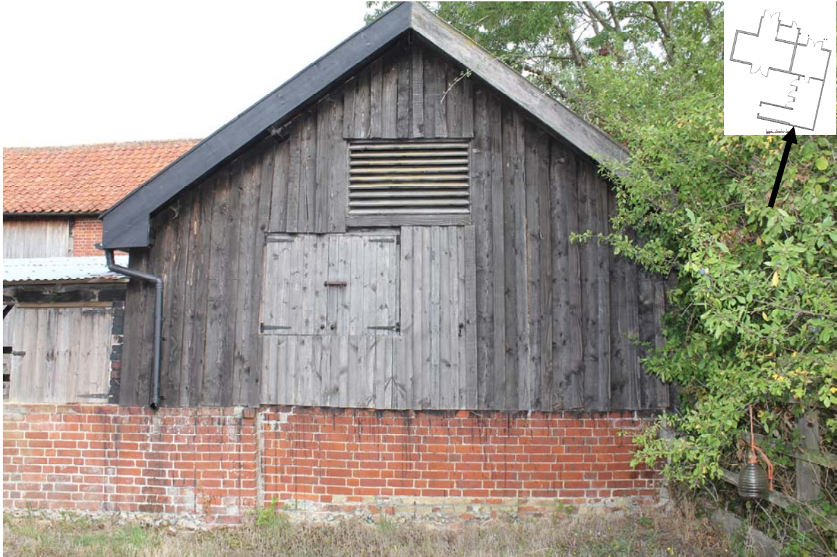
Fig. 31 Rear gable of east shelter shed - framing maybe later alteration as some rebuilding of the dwarf wall
