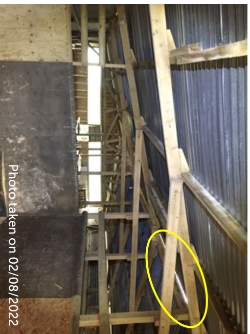
View looking south-east. Note the gap along the apex of the barn where roof sheeting overlapped
