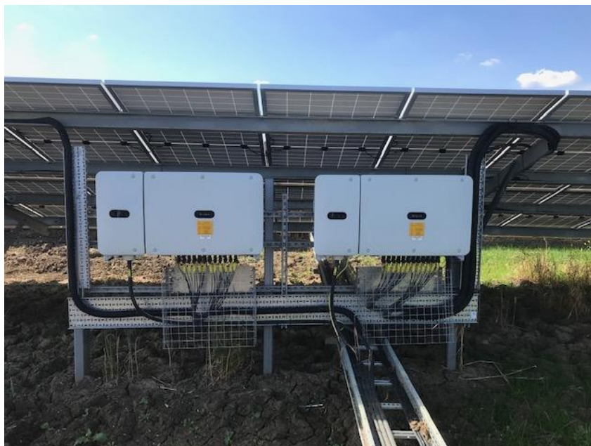
Figure 3: Inverters mounted onto the back of the solar arrays.
