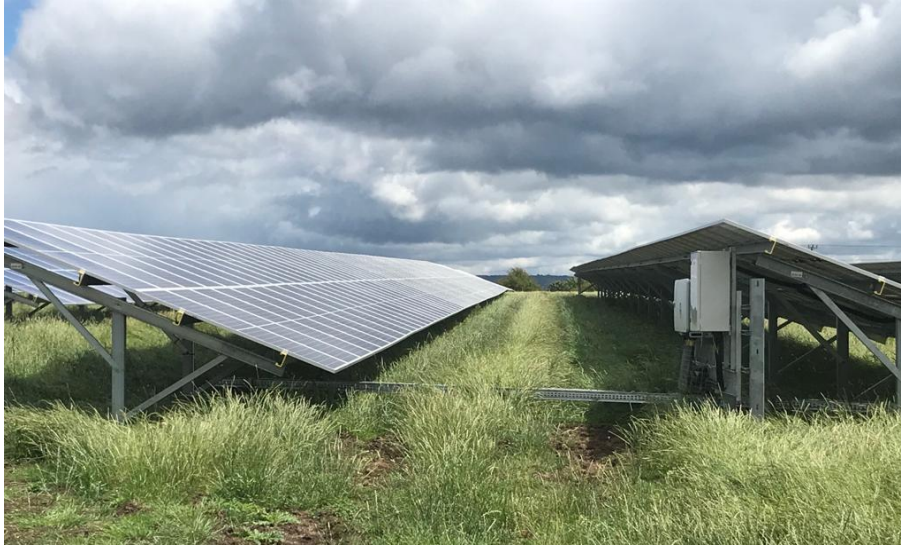
Figure 2: Example of rows of solar panels on mounting frames
