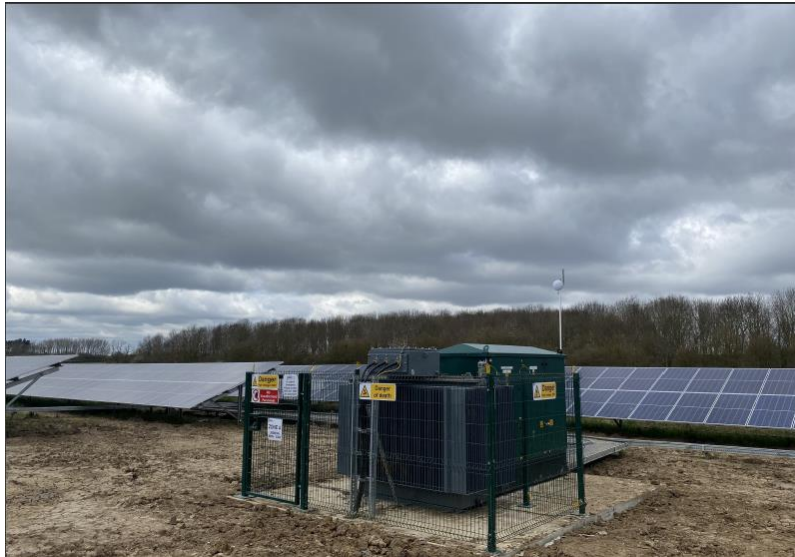
Figure 4: Typical LV Switchgear with Transformer
