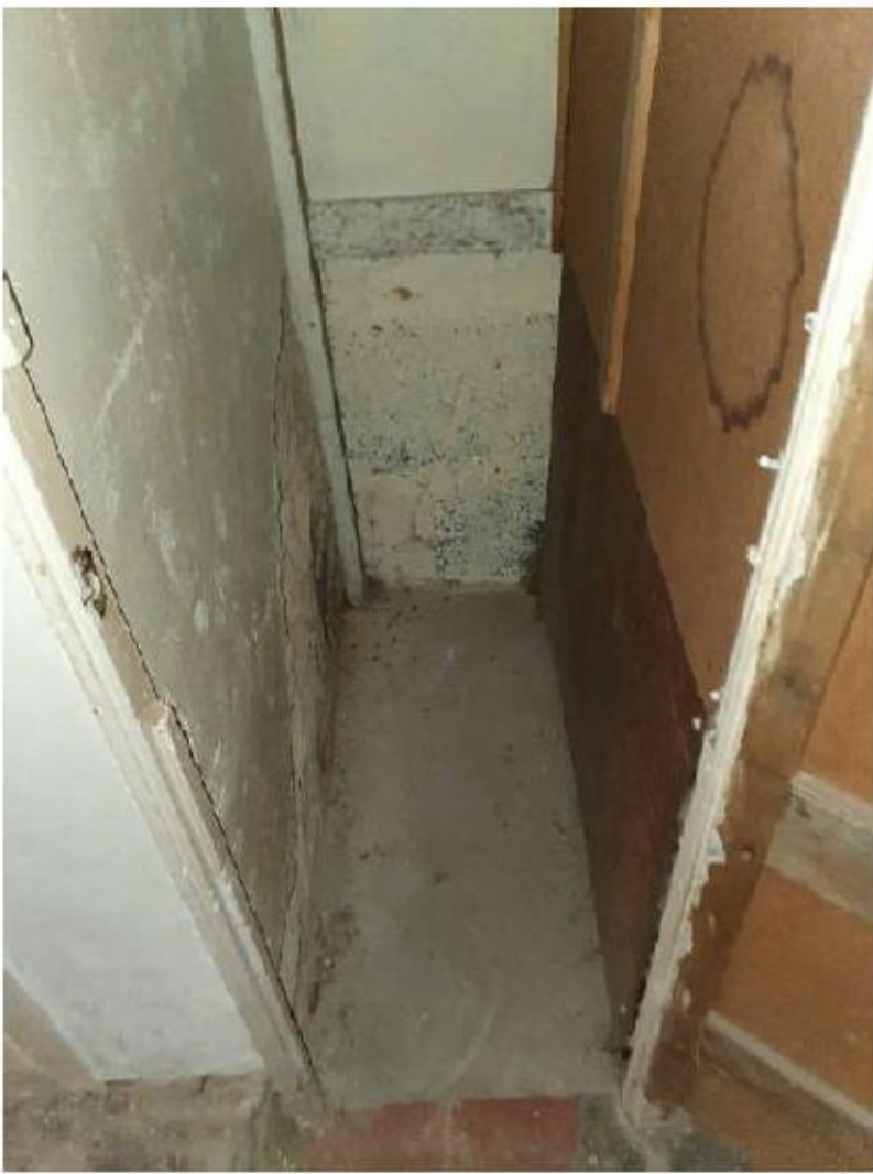
Evidence suggesting poor use of internal space
