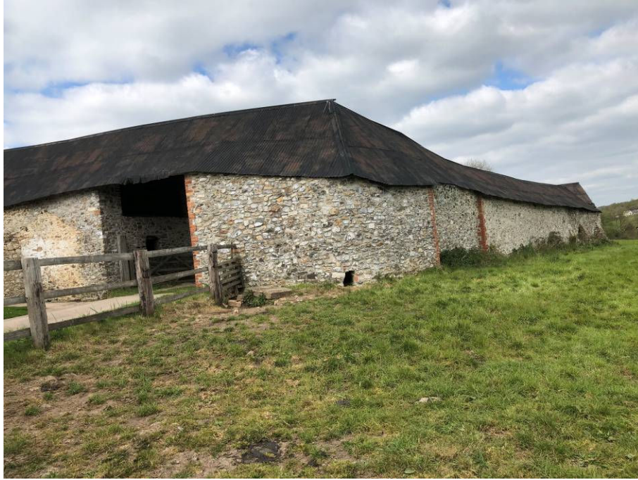
Figure 3 entrance to yard showing partly collapsed roof and repair.
