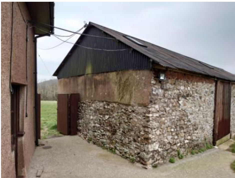
Fig.4 – Site Photo – View of NE barn and end wall for location of new pedestrian access door into proposed pump room.
