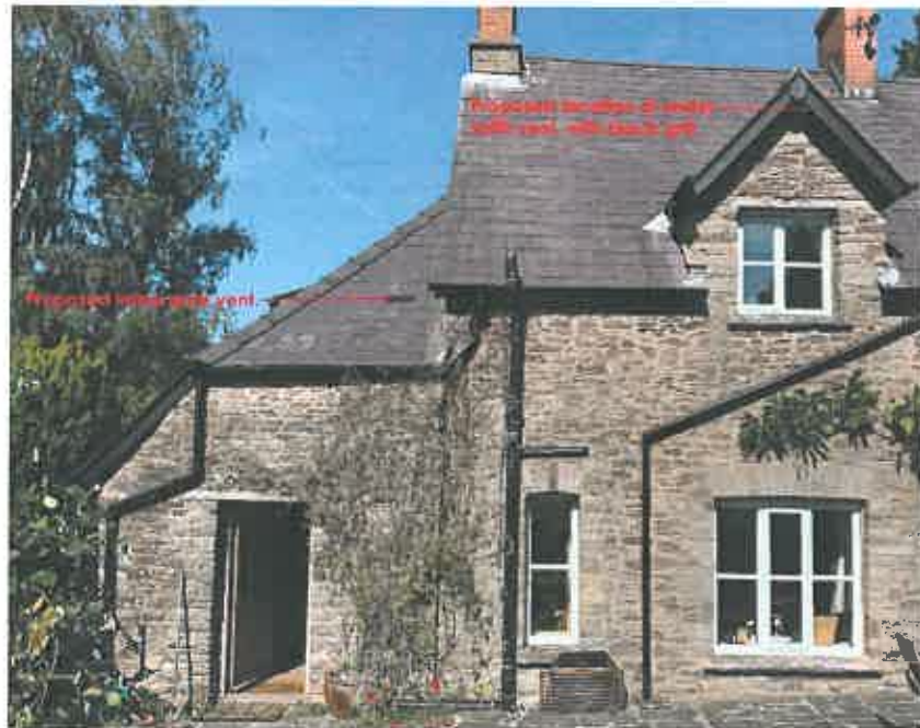
Inline slate vent in roof of cellar
