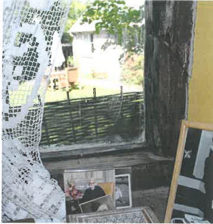
Scarfed section evident internally
