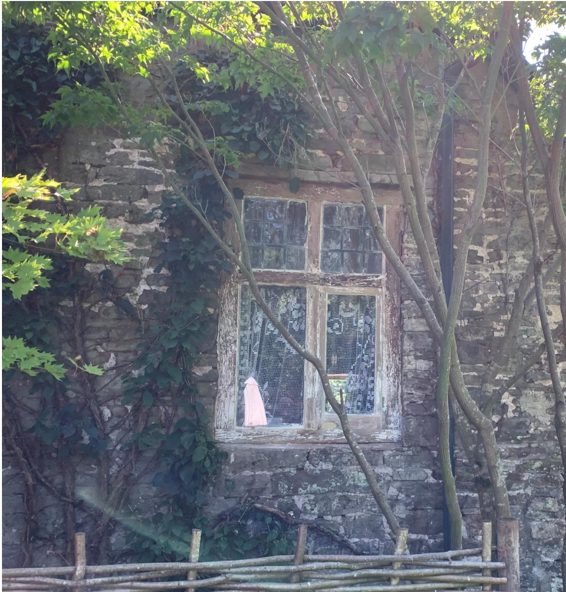
Photo of the north elevation with the late C17 early C18 window
