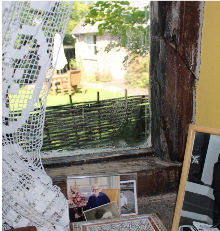
Scarfed section evident internally
