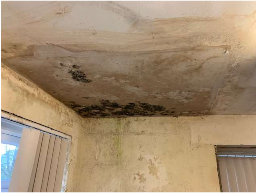
Damp stained ceiling
