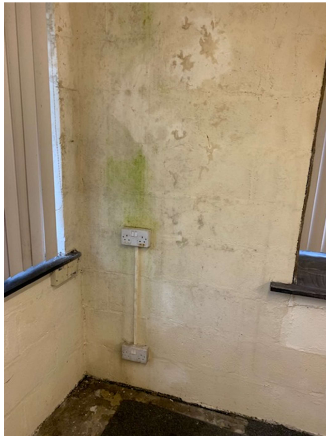
Damp stained wall within office
