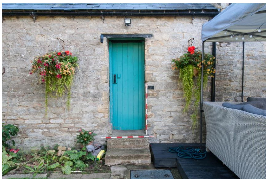
Figure 18 Doorway with brick surround inserted into the stone wall of the west wall
