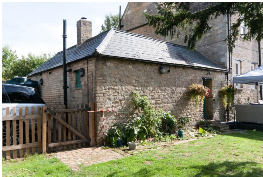
Figure 17 The join of the north and west ranges showing change between stone and brick walls
