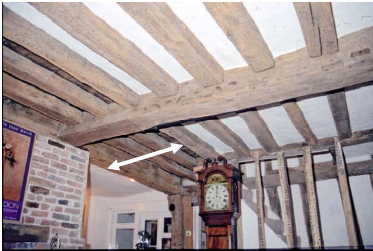
Undershot crosspassage and service end of 47 Castle Street, Saffron Walden. Open hall was to the left, now with inserted chimney but no mortices for partition between undershot crosspassage (indicated by arrow) and service room.
