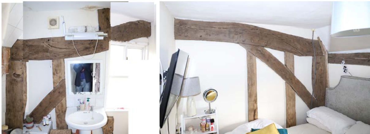
Fig 14: West face of cambered tiebeam over east gable EE' - north end to the left, south to the right
