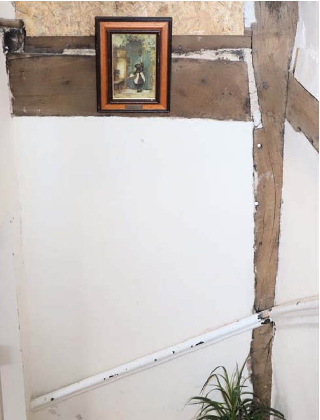
Fig 8: East face of principal post C' with pegs for an arched headed door
