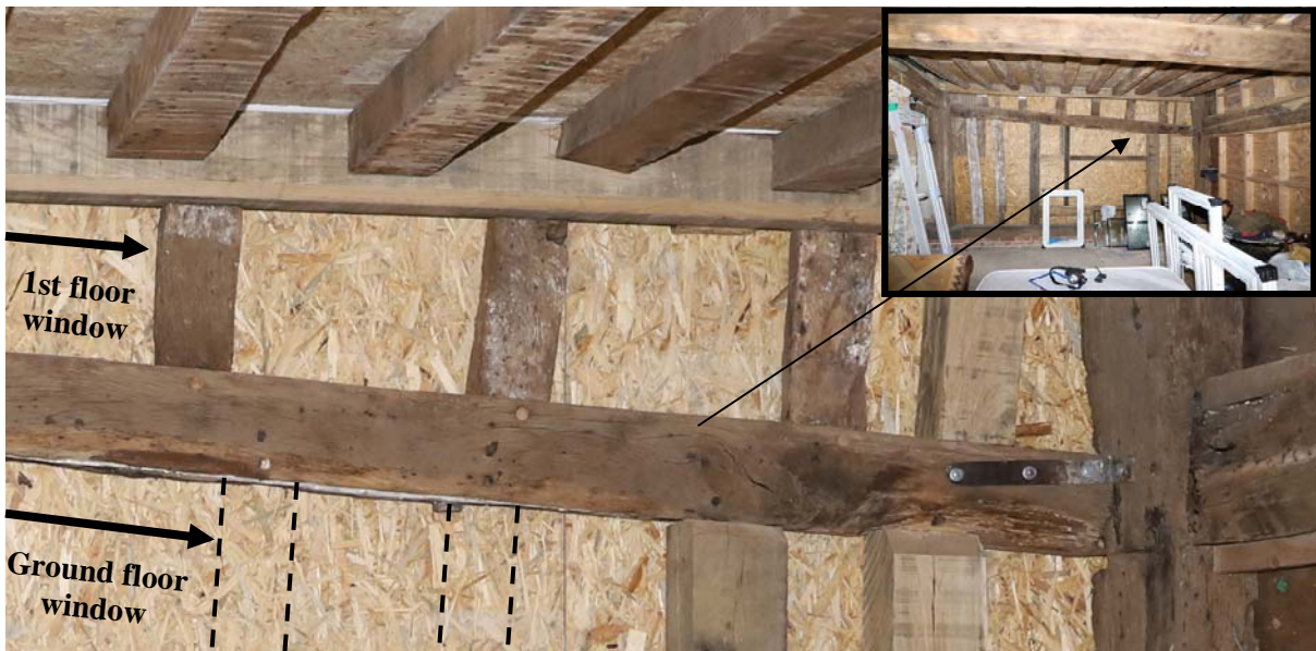
Fig 19: Midrail in front wall of parlour where pegs & the surviving lower stubs of the first floor studs show that the first floor window was not directly over the ground floor window
