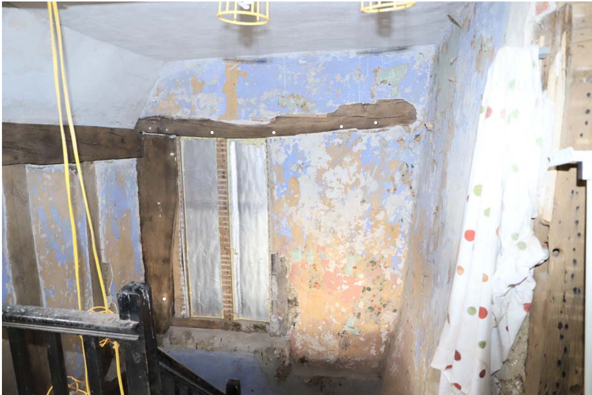
Fig 16: West face of north end tiebeam and principal post C' in chimney bay - pegs picked out in white
