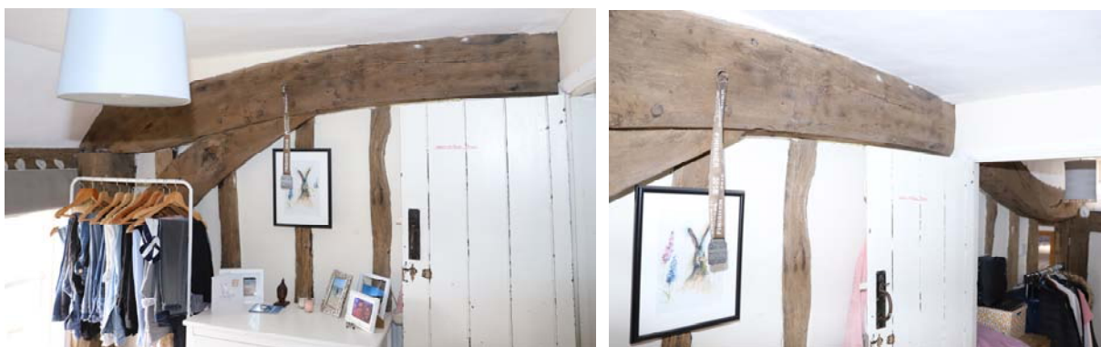
Fig 15: West face of tiebeam on truss DD' - south end to the left and north to the right
