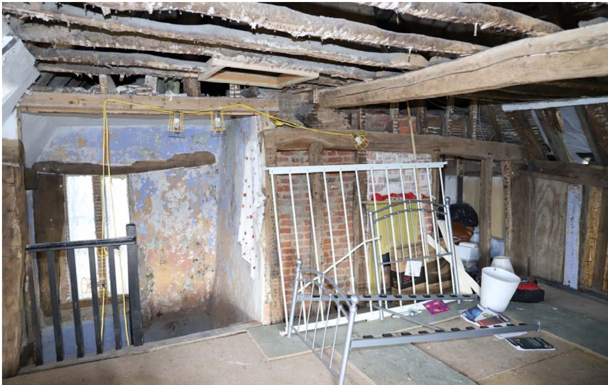
Fig 20: East side of parlour chamber (Victorian fireplace at right hand end of chimney stack)
