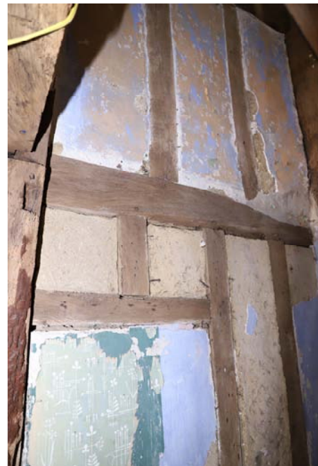
Fig 10: Rear wall of chimney bay showing ground and first floor studs (blocked door is a later insertion)
