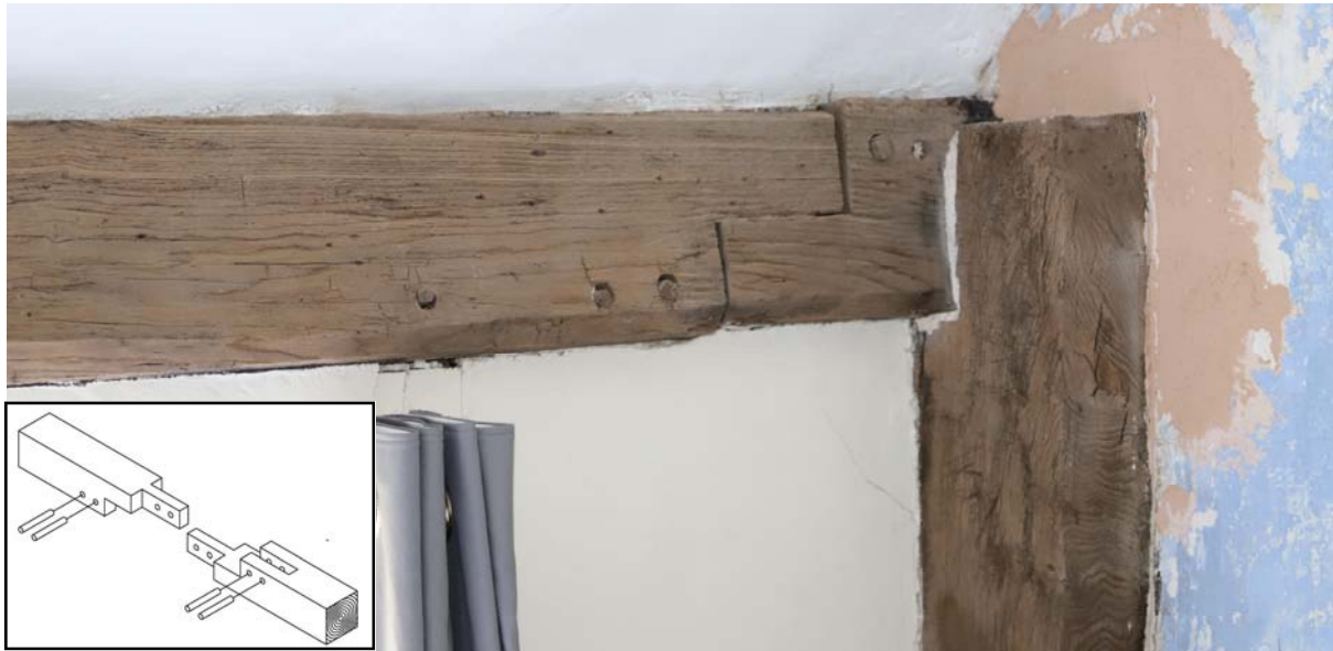
Fig 26: Edged halved and bridled scarf joint in south front wall east of post C.
