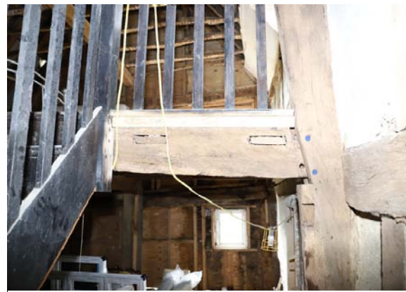
Fig 13: Looking west at east face of bridging joist BB' showing mortices for joists over lobby in chimney bay on north side of chimney stack
