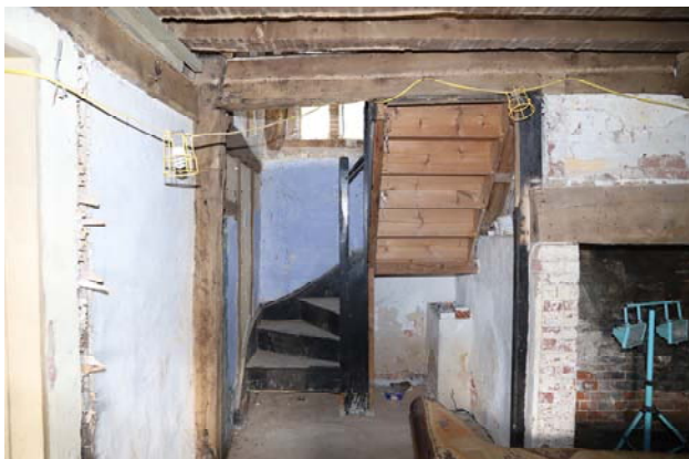
Fig 12: Stairs now in lobby on north side of fireplace in the chimney bay
