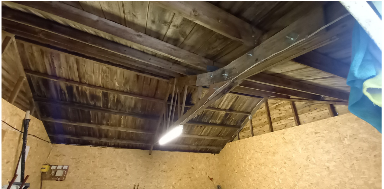
Figure 4 – Internal view of existing garage showing temporary repairs and water ingress
