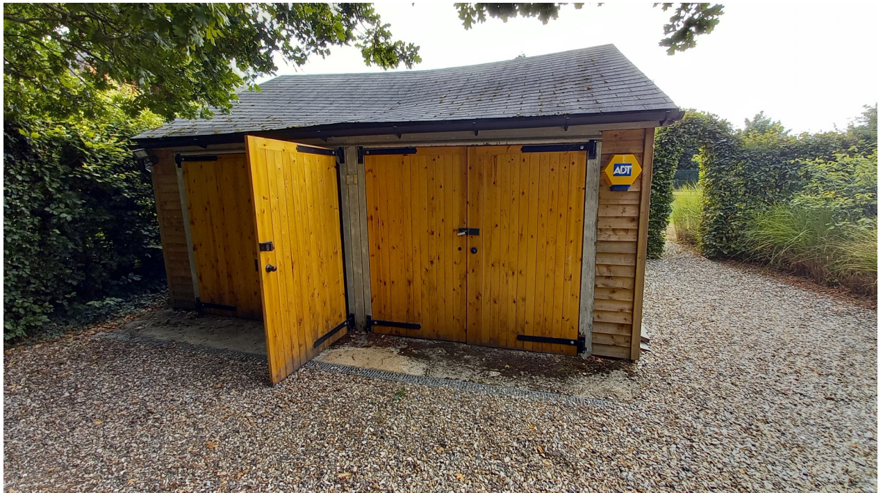
Figure 5 – External view of existing garage showing deflection of roof through truss collapse
