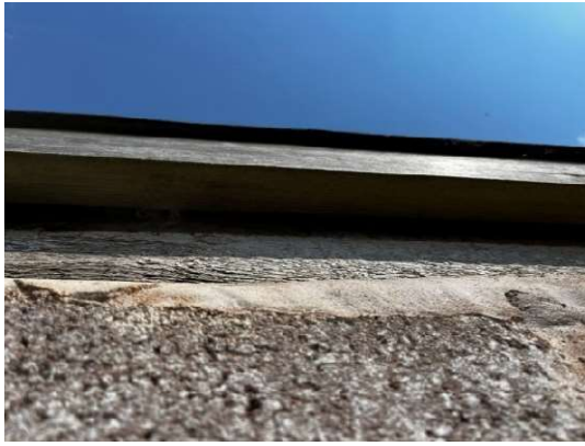
Plate 8. Gaps under the wooden fascia along the western elevation
