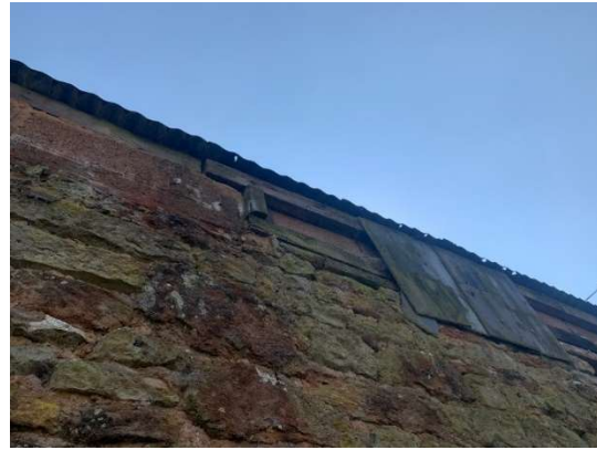
Plate 9. Gaps behind the hanging tiles and crevices within the stonework along the northern elevation
