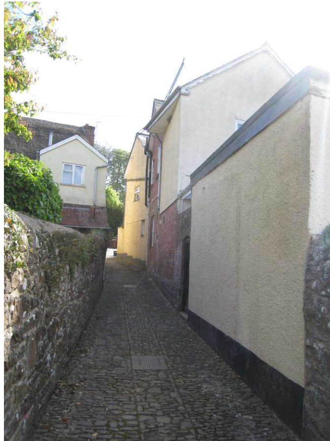
North west end of apartment where a proposed new window is to be inserted
