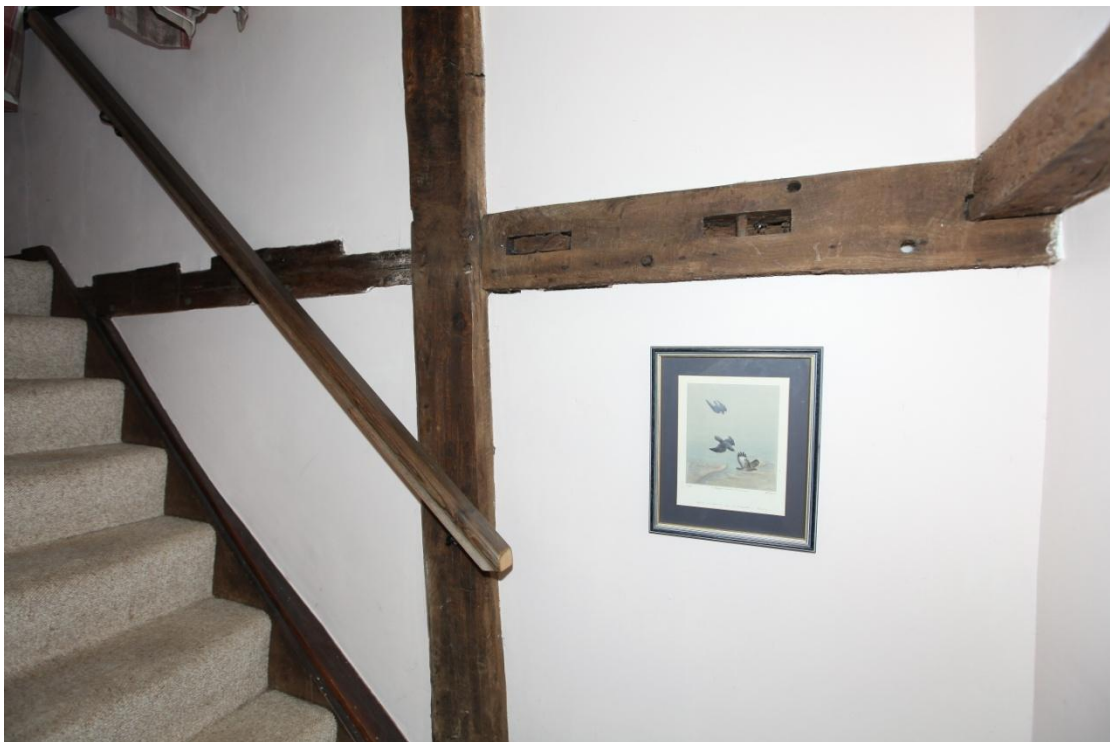
Illus. 18. The exposed framing of the original facade against the modern stair showing mortices for flat-sectioned joists in the mid-rails which are tenoned to the central storey post. These joists were removed to accommodate the stair which probably lay on the other side of the chimney initially.
