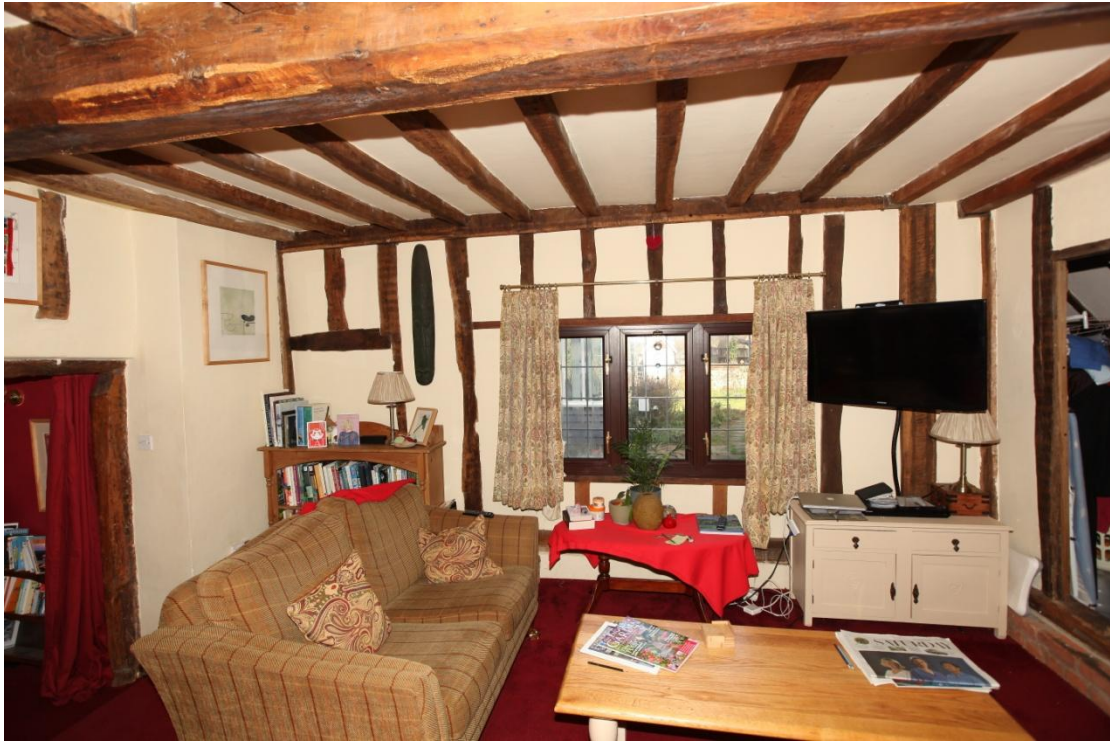
Illus. 11. The original north-eastern facade of the sitting room (2) with its modern PVC window and the blocked secondary door to the former lean-to addition on the left. The tall-sectioned ceiling joists are tenoned to the mid-rail, with no evidence of flat-sectioned predecessors, and the rail contains pegged mortices for three studs on each side of a central window. The narrow studs above the present window are later replacements.
