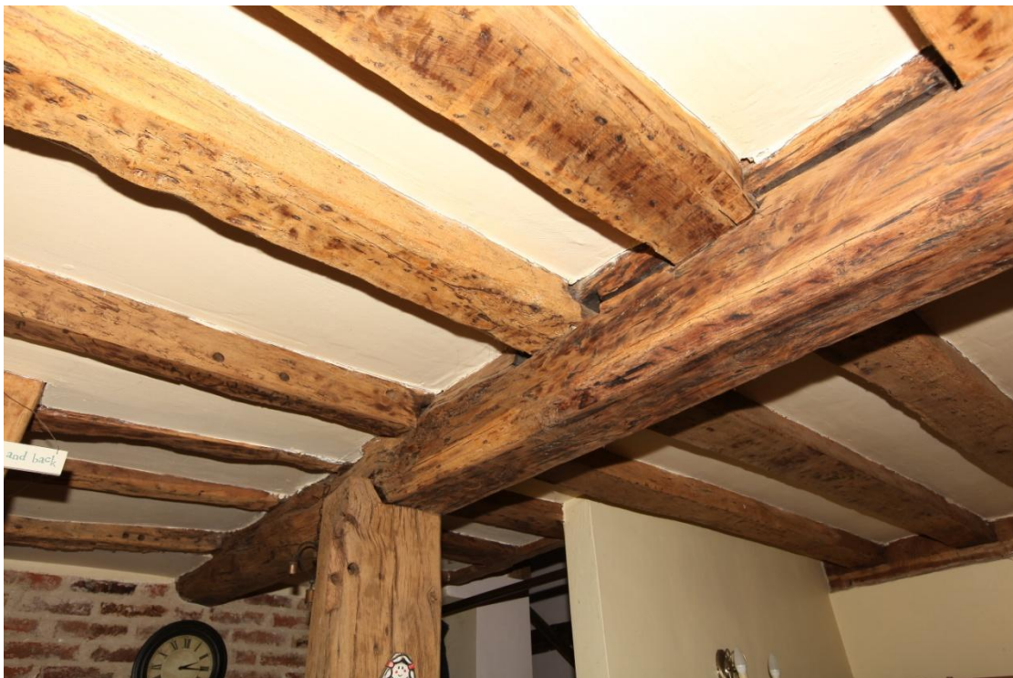
Illus. 16. The ceiling of the kitchen (3) where the joists are also tenoned to the front mid-rail to the north-east and lodged on the rear but consist entirely of flat-sectioned timbers. The four joists to the left in this image have been replaced with re-used timber and may indicate the position of an earlier stair. Exposed framing had ceased to be fashionable by the mid-17 th century and these timbers would have been hidden by insulating plaster initially.
