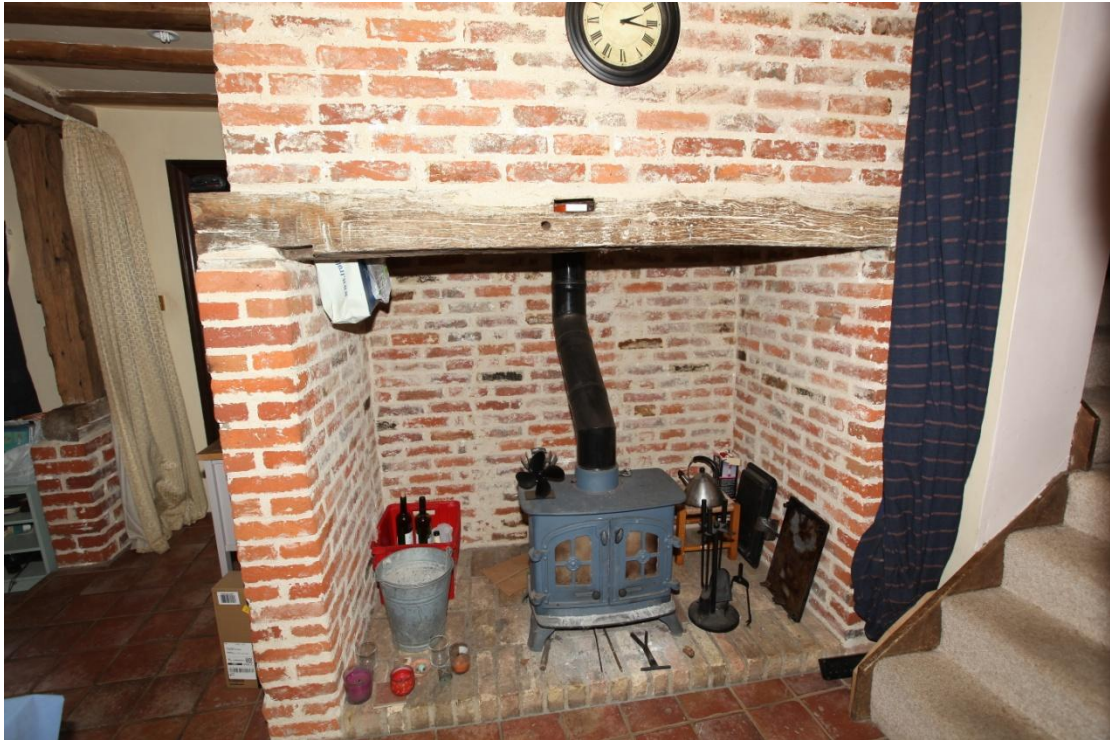
Illus. 17. The fireplace facing the kitchen (3) with the foot of the 1980s staircase on the right and the modern entrance porch to the left. The timber lintel and bricks are re-used, like those of the sitting room (2), and the entire chimney appears to have been rebuilt as part of the 1980s refurbishment. The flue above consists entirely of modern Fletton bricks laid in cement mortar where visible in the roof void.
