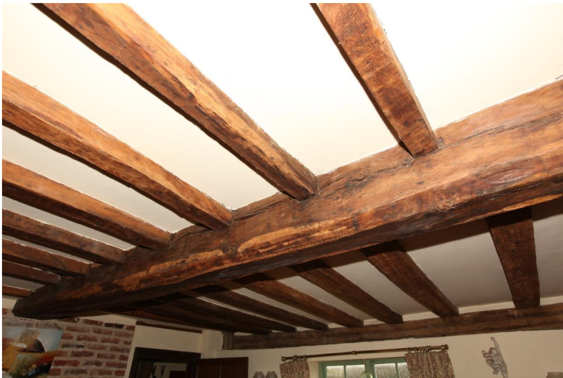
Illus. 14. The opposite side of the axial joist in the sitting room (1) showing the tall-sectioned common joists with no mortices for flat-sectioned predecessors. The mid-rail in the rear lacks joist mortices but is otherwise identical that of the original facade with three pegged stud mortices flanking a central gap for a window. It is highly unusual to find two entirely different forms of carpentry in the same structure.
