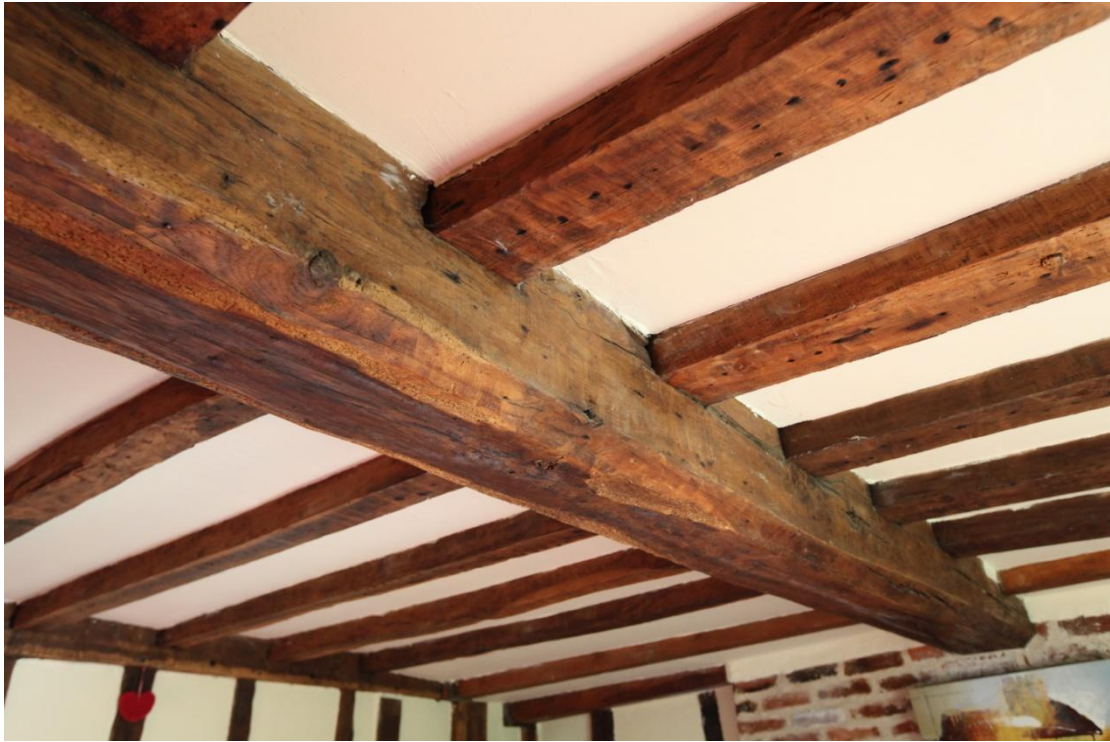
Illus. 13. The ceiling of the sitting room (1) from the north-west showing its unusual combination of narrow, tall-sectioned joists to the left of the axial joist – all tenoned to the mid-rail – and flat-sectioned joists on the right which are lodged on the mid-rail.
