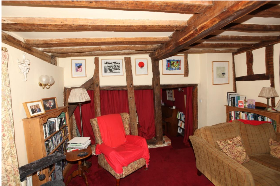
Illus. 9. The north-western wall of the sitting room (2) in the two-storied extension showing the much lower ceiling of the earlier parlour beyond. The blocked door on the right opened into the demolished lean-to shown in figure 7 and is a later insertion.
