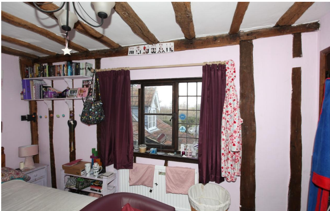
Illus. 20. The early-20 th century leaded-light casement window in the original north-eastern facade of the bedroom above the sitting room (2). The ostensibly original ceiling joists on the first floor consist largely of re-used timbers, as do the small areas of exposed wall framing. The rails supporting the joists lie approximately 12 inches below the chamfered roof-plates to create low vertical walls on the attic storey and the base of a jowled corner post is visible to the left.
