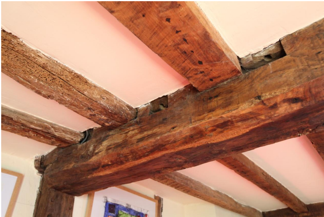
Illus. 12. A detail from the south-west of the axial ceiling joist in the sitting room (2) showing pegged mortices for original smaller, tall-sectioned joists matching those visible in the rear. The large, flat-sectioned joists in illustration 13 are either replacements or more probably re-used timbers intended to be hidden by plaster.
