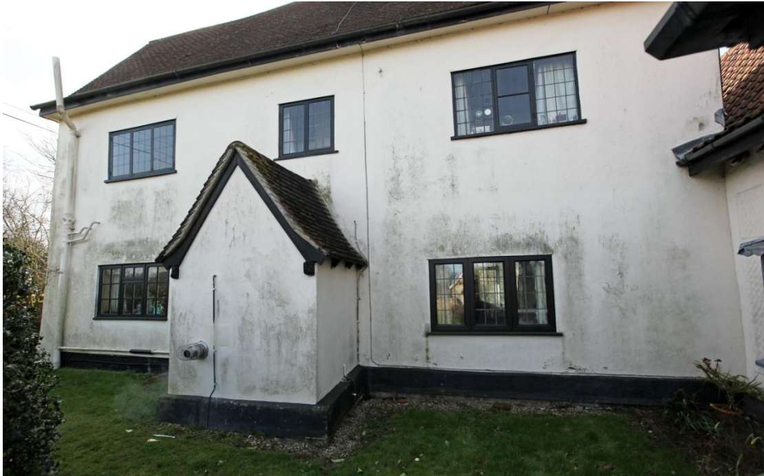
Illus. 3. The north-eastern facade of the extension with its ostensibly original timber-framed entrance porch. Two dormer windows have been removed from this elevation since 1964 and both ground-floor windows replaced (the right-hand example in PVC). The only window that survives from 1938 is the right-hand example on the upper storey which replicates the style of the 18 th century but dates from the early-20 th . The small central window was inserted between 1938 and 1964 and is identical to its larger counterpart on the left.
