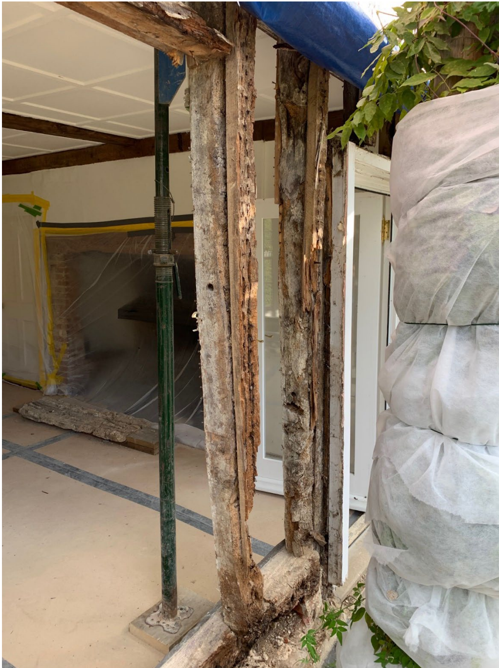
Sitting Room – South Elevation (note removed and stored wattle & daub panel in front of fireplace)
