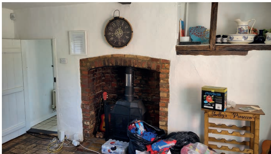
Large internal fireplace. Wanting to be retained as a key feature in the design.
