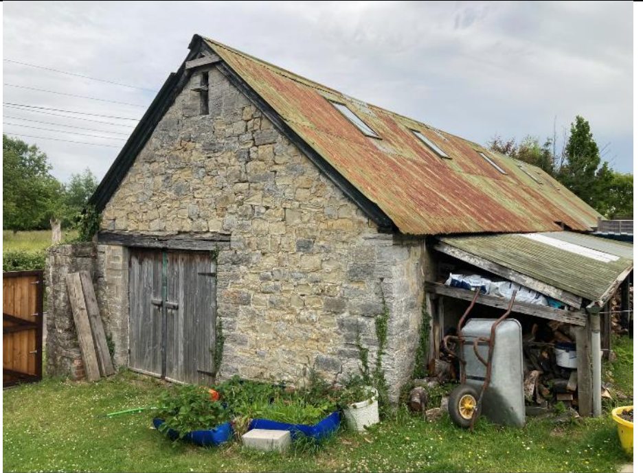
Photo 1: Showing the southern and western elevation of the building B1 and the small lean-to off the southern elevation.
