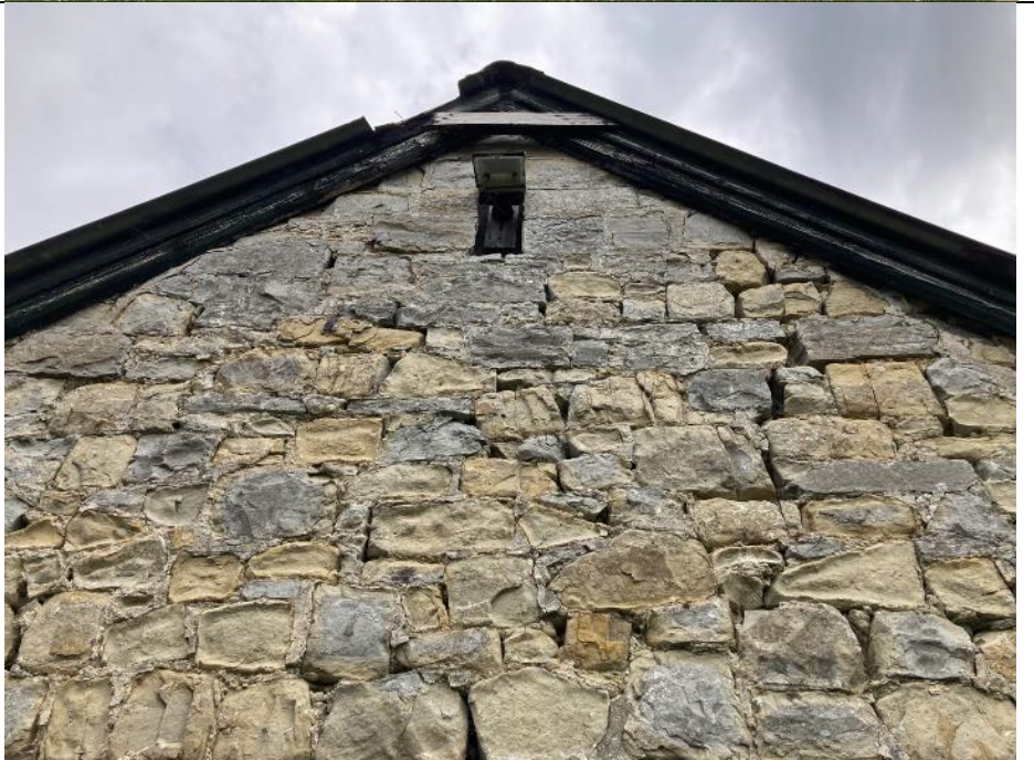
Photo 2: Showing the gaps under the fascia of the western gable end as well as the gap in the stonework at the apex and across the areas of missing mortar.
