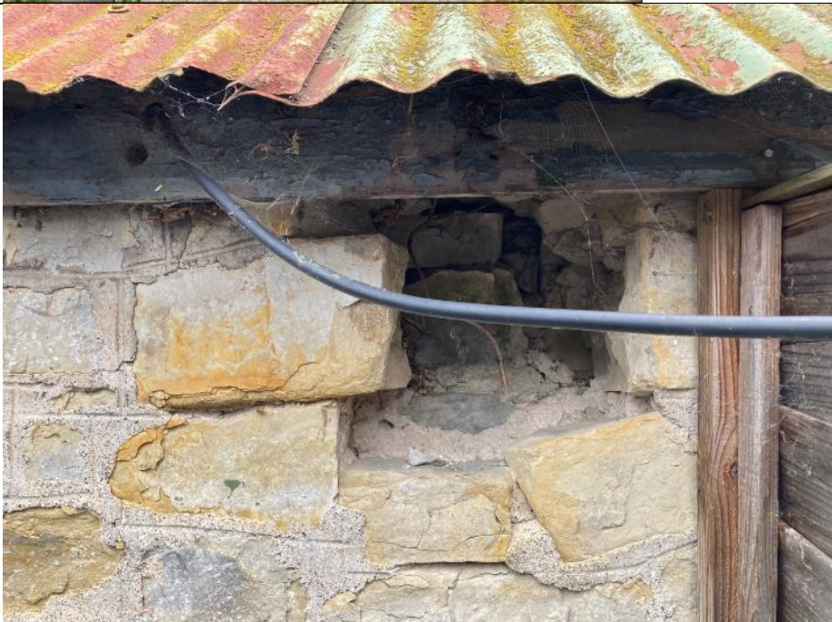
Photo 4: Showing the area of missing stonework at the eastern end of the southern elevation.
