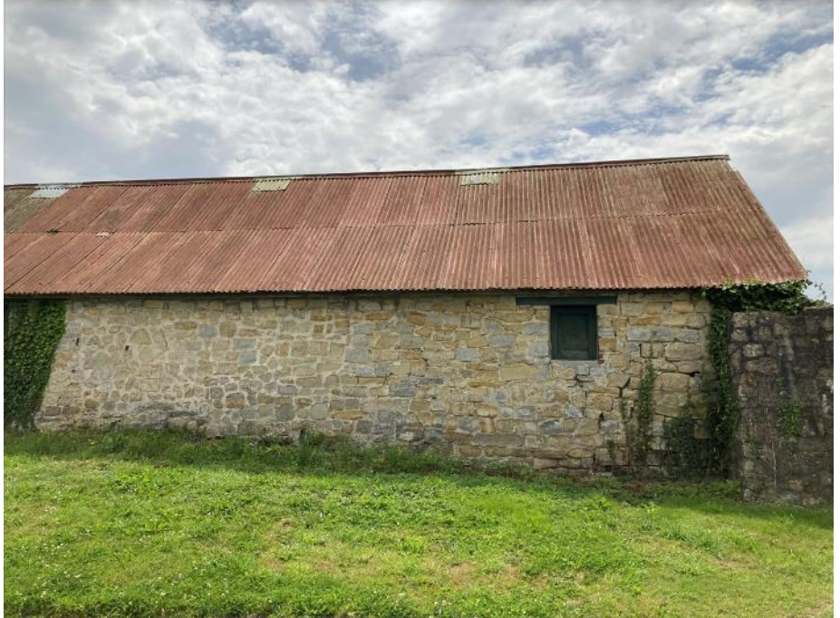
Photo 5: Showing the northern elevation of B1 with gaps in the stonework at the western end of the wall.
