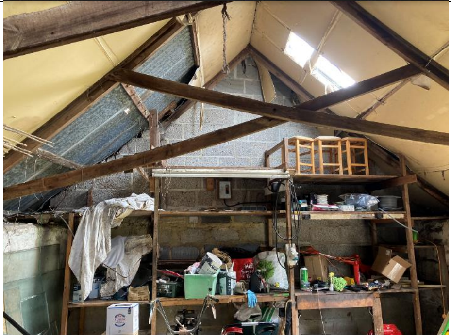
Photo 8: Looking at the eastern gable end showing the gaps along the wall top.
