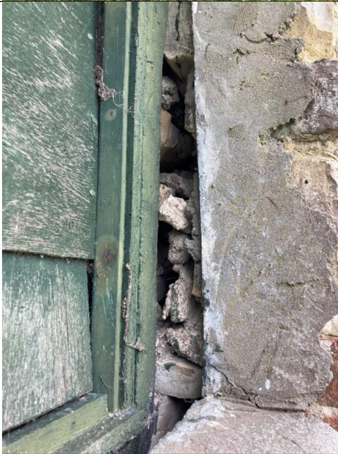
Photo 6: Showing the gaps in the stonework around the wooden window on the northern elevation of B1.
