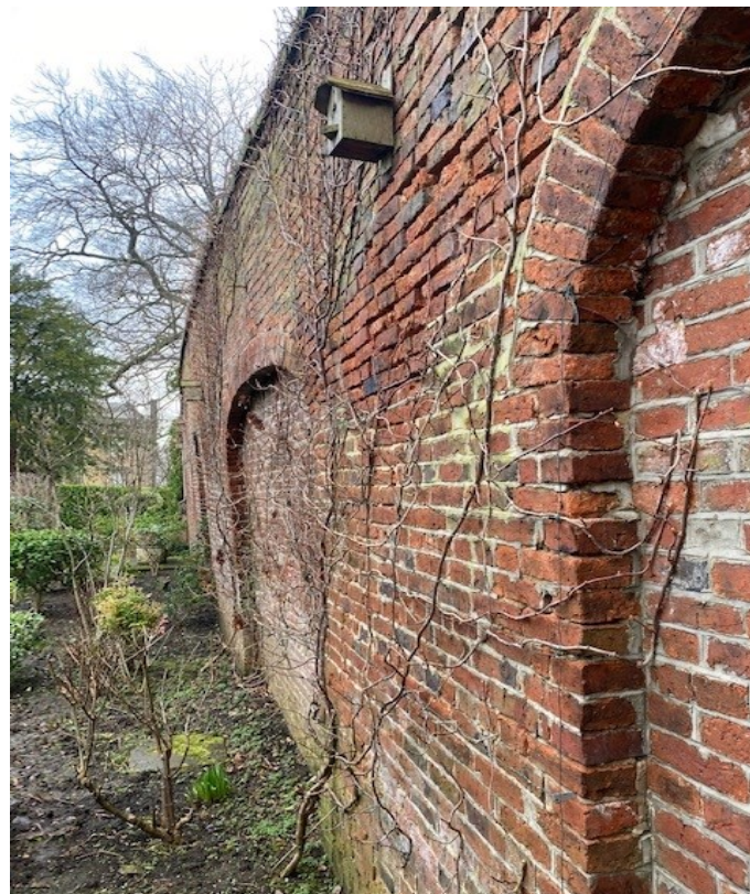
Photo A1.4 : There are widespread signs of erosion to the brickwork.
