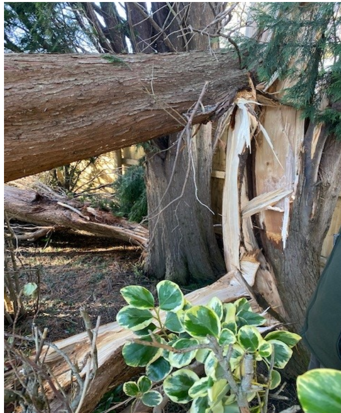
Photo A1.8 : Close-up of tree trunks at Bretton Lodge, split by Storm Eunice.
