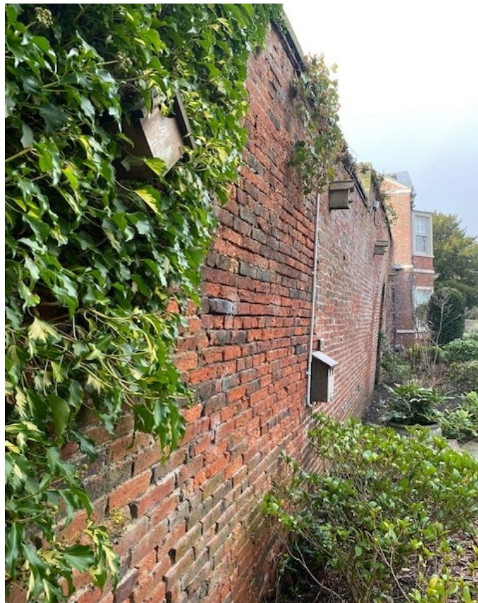
Photo A1.2 : The wall has a pronounced lean of up to approx. 600mm to the north.
