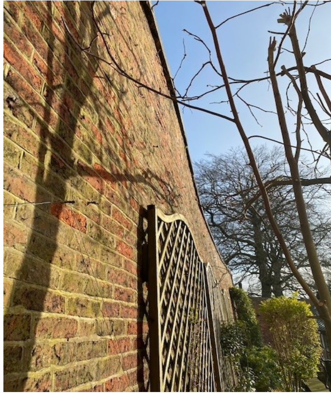
Photo A1.3 : The head of the wall has distorted into a smooth curve over approx. three quarters of its length.
