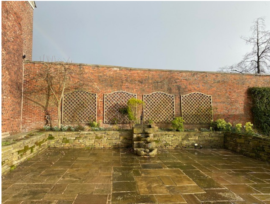
Photo A1.5 : There are no signs of physical impact or abrasion to the south face of the wall.
