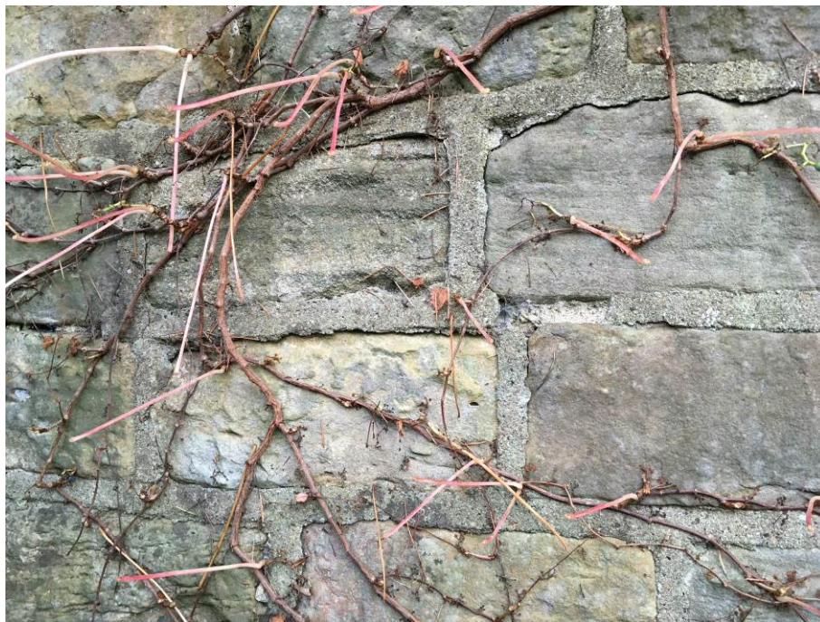
Photo A1.10 : Cracking and localised loss of pointing to the western coursed sandstone face of the wall. NB fracturing of individual masonry units does not appear to have occurred.
