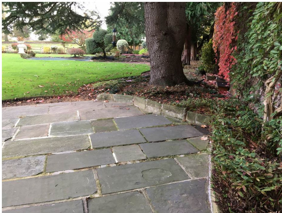
Photo A1.12 : The sandstone paving to the patio has lifted slightly, resulting in the loosening of pointing.
