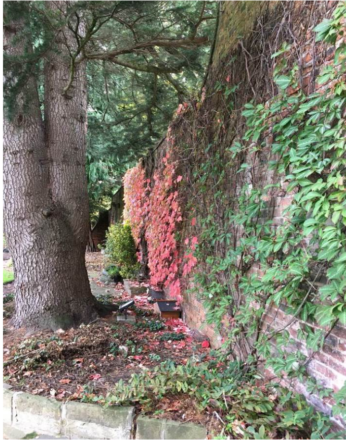
Photo A1.11 : There is a slight westward lean to the head of the wall opposite to the tree, estimated visually to be approx. 150mm.
