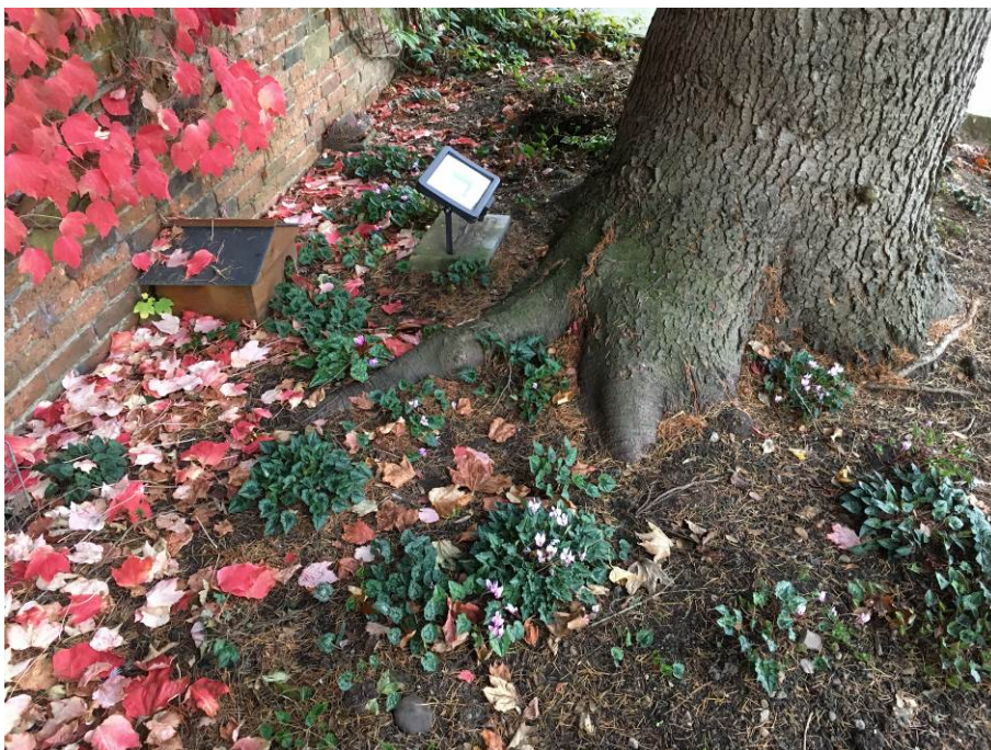
Photo A1.8 : Slight lifting of major roots to the south and west of the tree, with slight resultant lift in the bed joint coursing of the adjacent estate wall.
